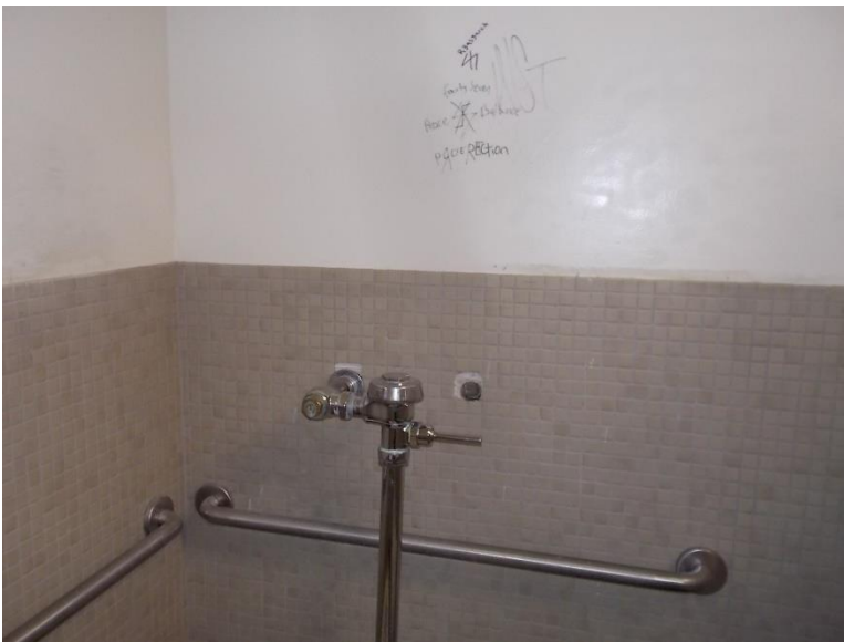
A17. Men's Restroom accessible stall; ceramic wall finishes have holes, and graffiti on wall finish.
