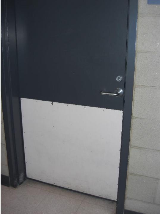
D1. First floor equipment room door. Door protection attached to door.
