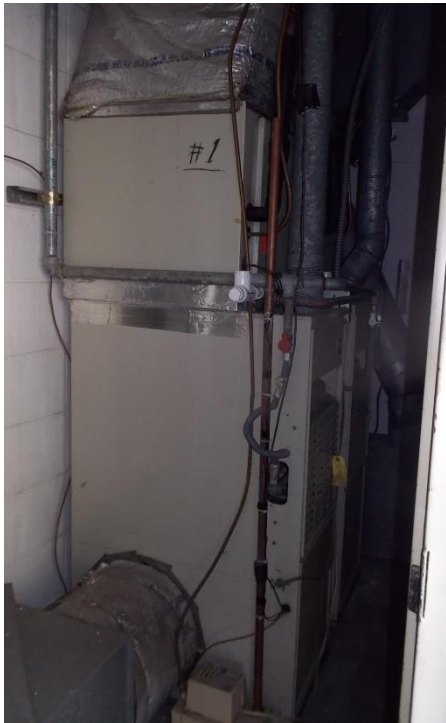
M1. Gas fired forced air heating units in mechanical closet, typical.
