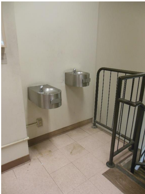
DF4. Top of Stairwell 147; non-compliant hi-low drinking fountains.
