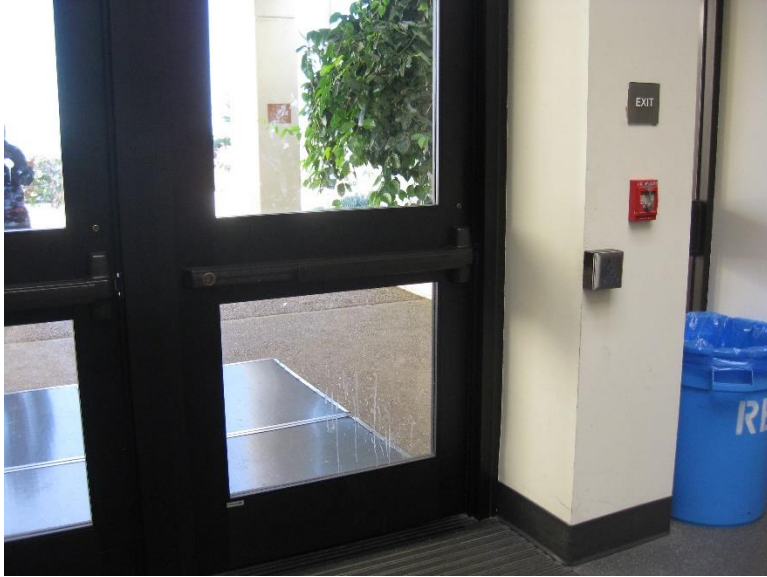
D5. Lobby main doors; non-compliant push-side clearance. Electronic door operator low level access button is required by code.
