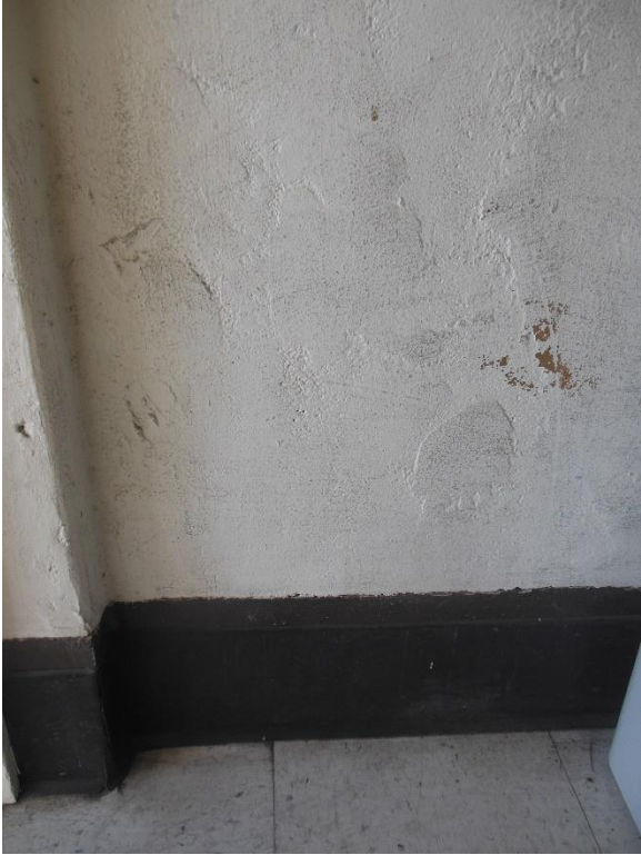
AI3. Office 11 foyer, plaster wall damage.
