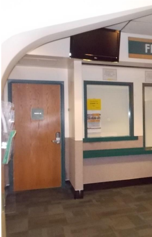
D4. Second floor office; pull-side clearance not met.
