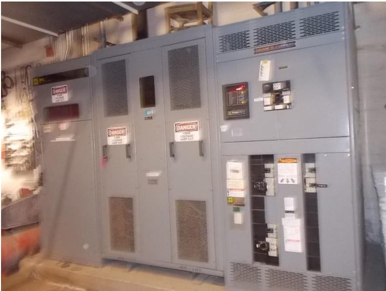
E2. Switchgear in basement.
