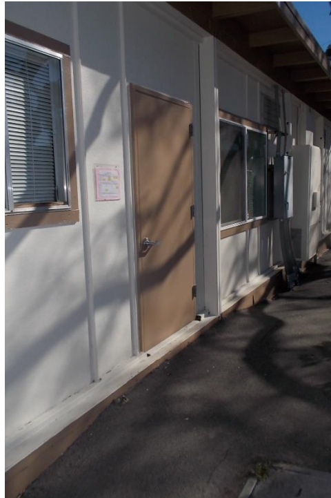
D2. Portable 22, excessive threshold height.
