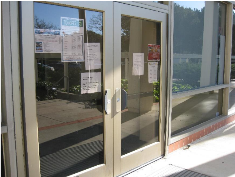
D2. North side entrance; ISA sign not installed.
