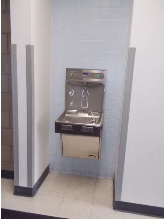
DF1. Bottle filling station/drinking fountain. Compliant maneuvering clearances are not provided.
