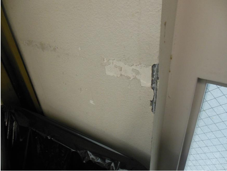
A3. Library vestibule; wall damage.
