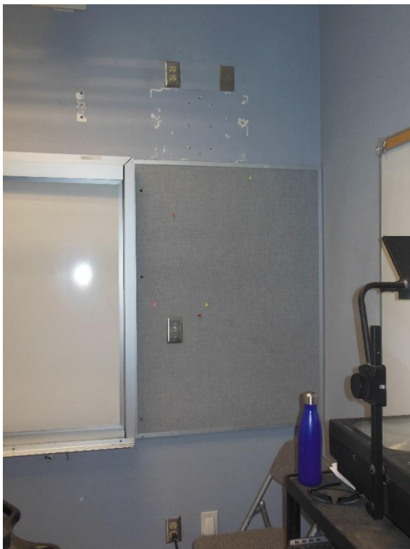
A6. Second floor classroom; wall repair damage.
