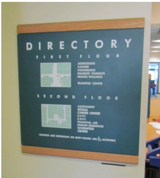
S2. Directory sign; no evacuation or other way finding signs are in the facility.
