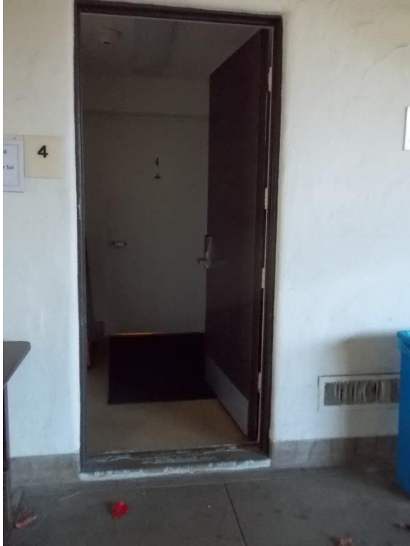
D6. Classroom 4, non-compliant threshold.
