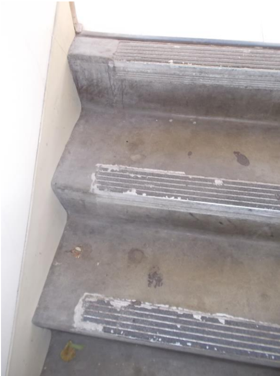
S1. Exterior stairs with non-compliant nosings.
