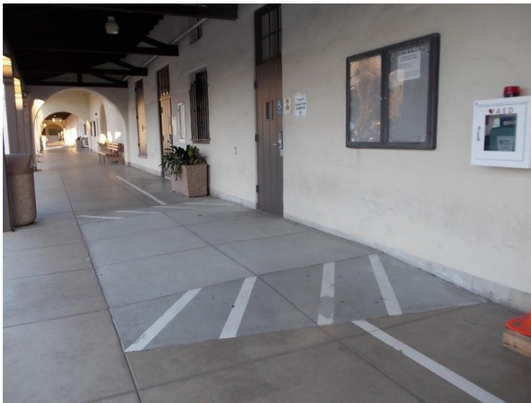
PT2. Exterior walkway; path of travel interrupted by ramp.
