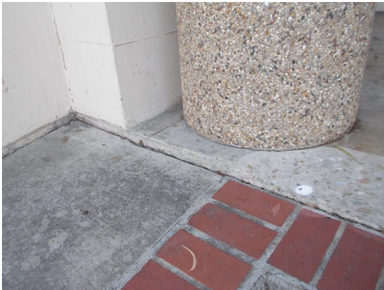
PT2. Non-compliant transition at East ramped entry.
