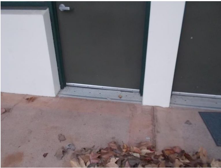
PT5. South side of building, Offices 115-117; door threshold slopes exceeds the ½" maximum height, and push-side dimensional clearances not provided.
