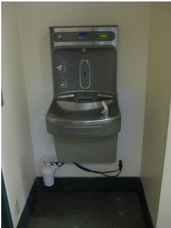
DF2. Bottle filling station/drinking fountain. Compliant maneuvering clearances not provided.
