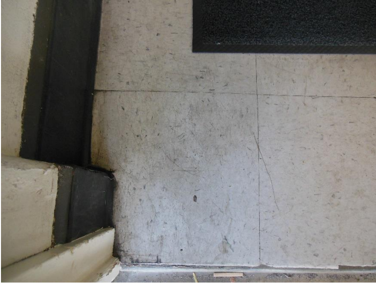
IF3. Office 11 foyer, VCT floor damage.
