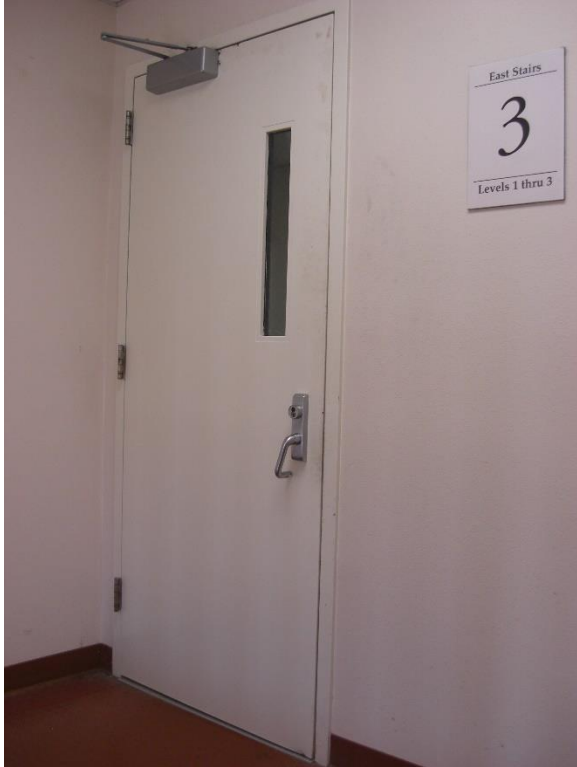
D3. Third floor stairwell door with damaged lever hardware.
