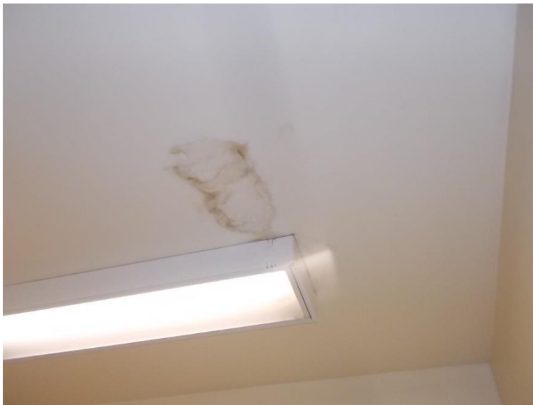
C5. Second floor Women's Restroom; gypsum board ceiling stained.
