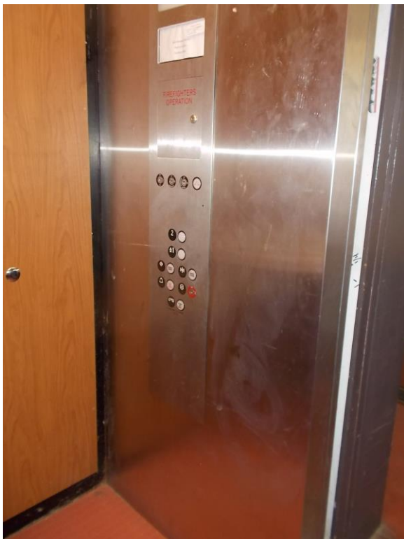
EV2. Elevator car interior.
