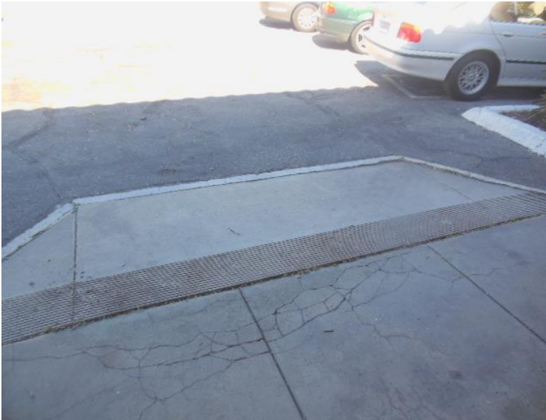
PT3. Curb ramp to parking lot; ramp cannot project into the path of cars, and are missing truncated domes. Concrete surface is cracked and degraded.
