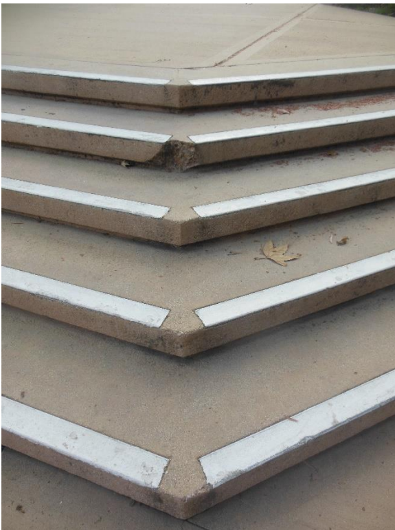
ST8. North side of building; exterior stair with damaged nosing, and missing handrail at change in stair direction.
