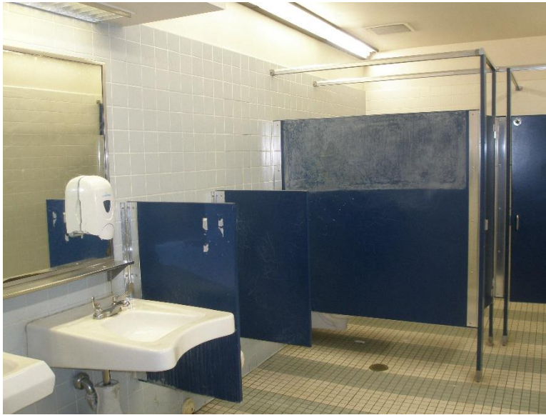
RR1. Mens restroom, accessible clear floor space not provided. Mirror and soap dispenser mounted above ADA compliant heights.
