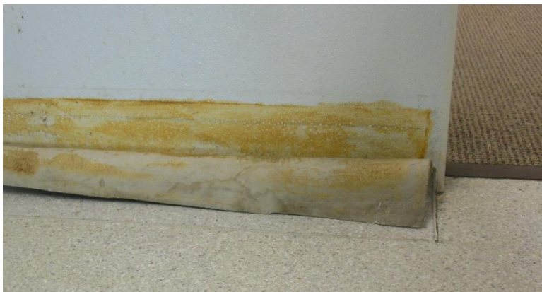
IF8. Library Café, upper floor; resilient cove base in very poor and unsanitary condition.
