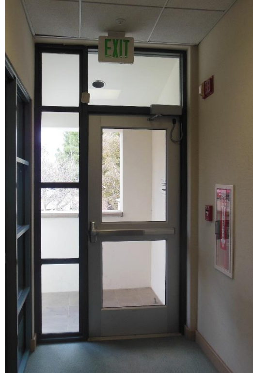
D5. Second floor corridor exit door. Tactile exit sign missing, and exit sign not illuminated.
