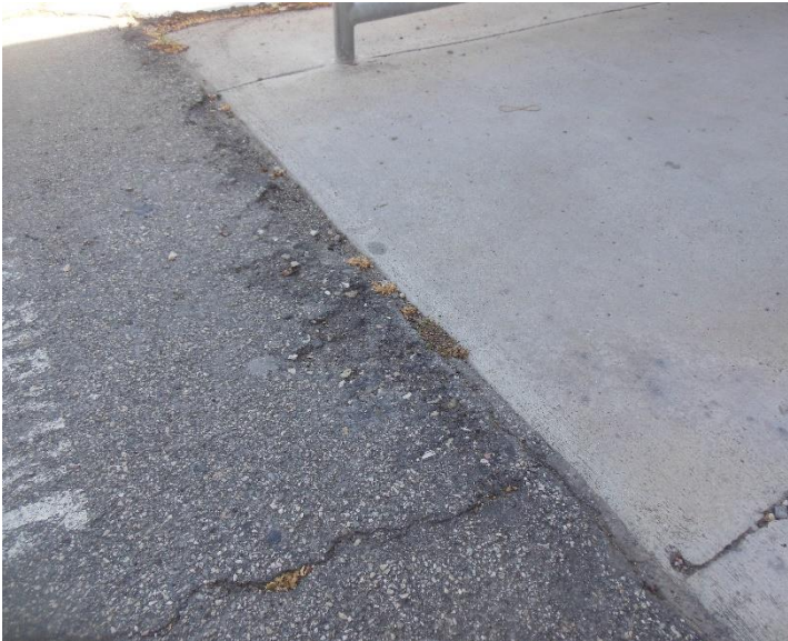
PT6. Landing at ramped walk to Men's restroom; abrupt change in level.
