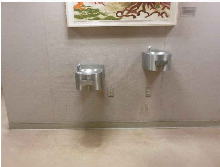
DF2. Second floor restrooms; non-compliant hi-low drinking fountains.
