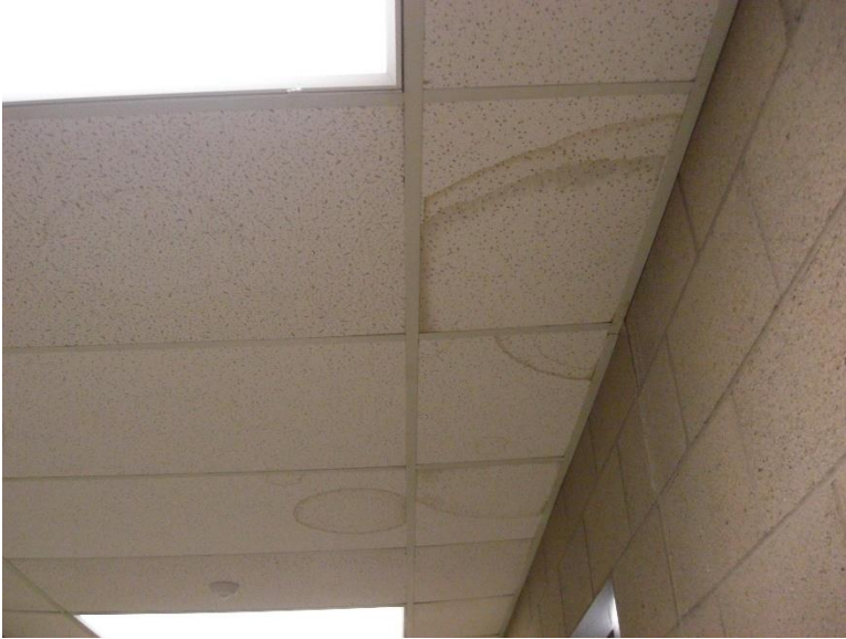
C1. First floor corridor ceiling system; water damaged.
