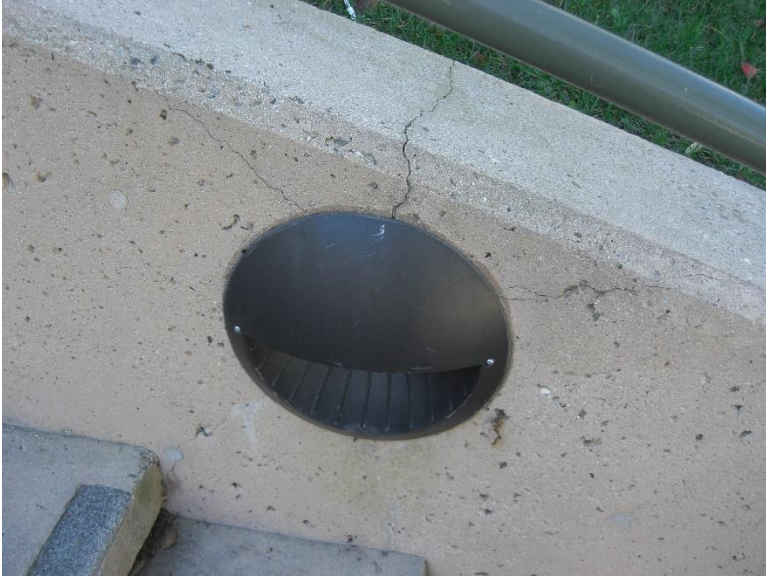
AE5. Cracked concrete wall at exterior stair.
