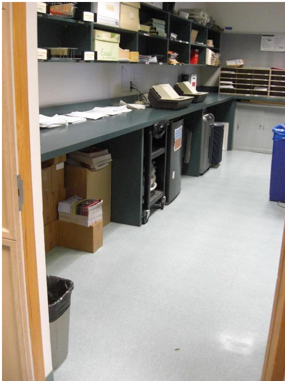
IF2. Second floor Workroom, damaged resilient floor.
