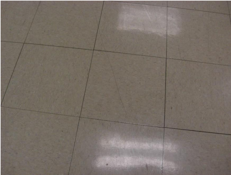
IF2. Second floor corridor; scratched/damaged VCT flooring.
