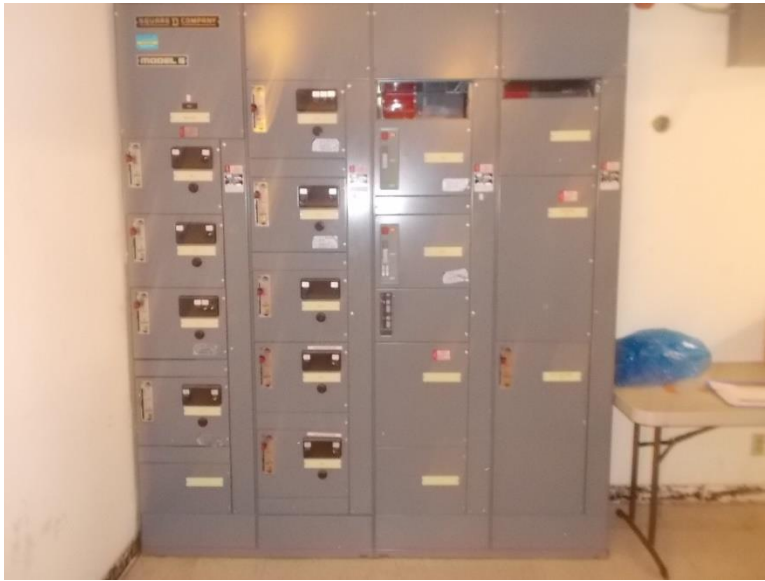
E1. Electrical equipment.
