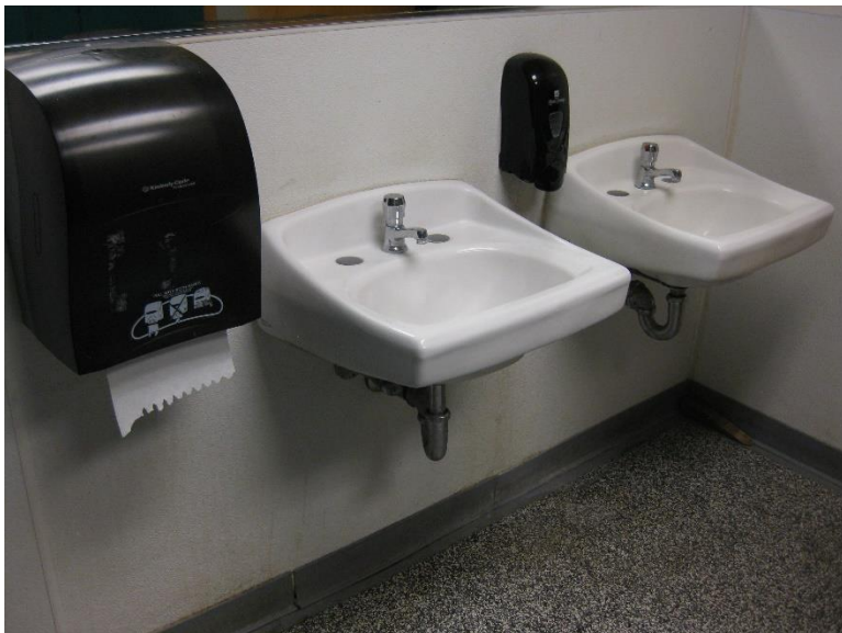
RR2. Sink does not provide paddle faucet fixture handles, knee protection is not provided at under sink plumbing traps.
