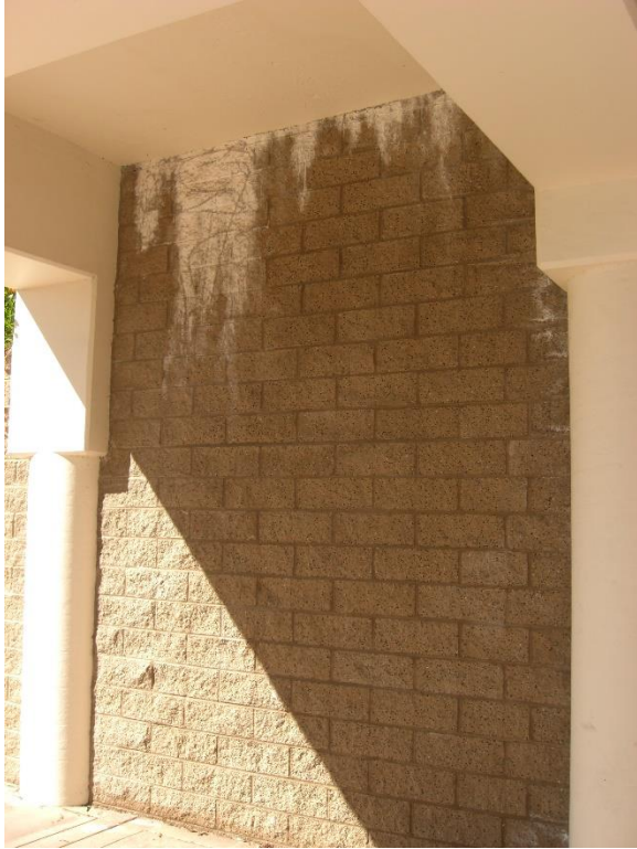
AE3. First floor CMU wall under overhang with efflorescence (white mineral deposits) from water intrusion above.
