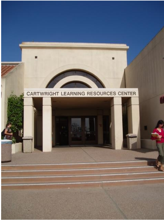
PT3. Main entrance, south side. Intermediate handrail at stairs required.
