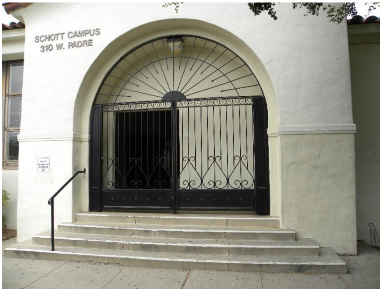
D1. Entrance from west side of site; missing handrails on right.
