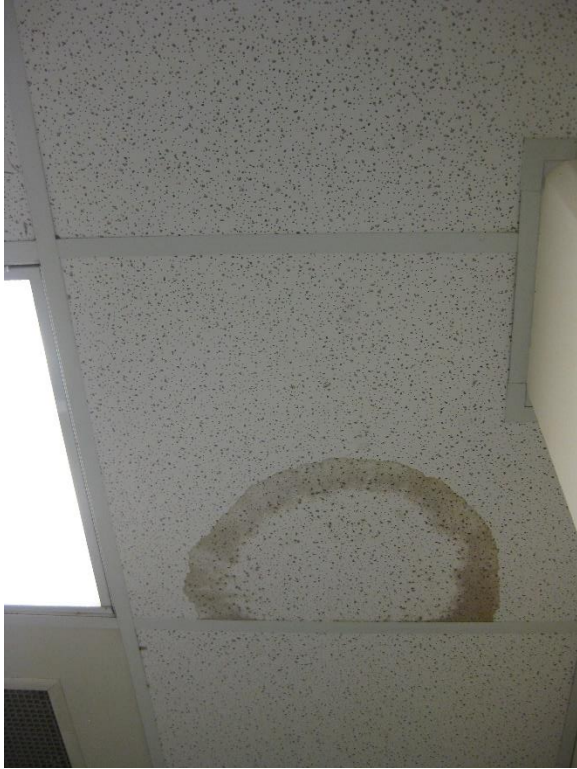
C4. Suspended ceiling tile; stained.
