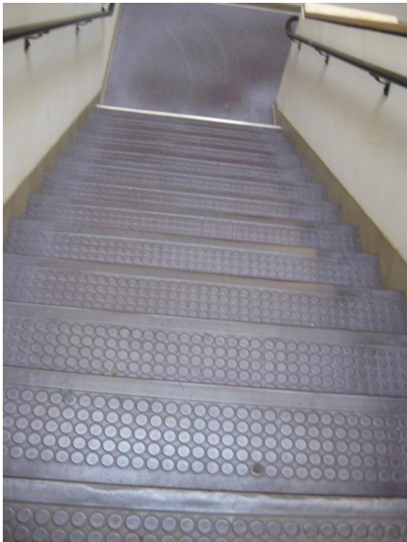
ST2. Library interior stairs; upper and lower visual warning stripes missing at stair nosings. Rubber treads worn and damaged.
