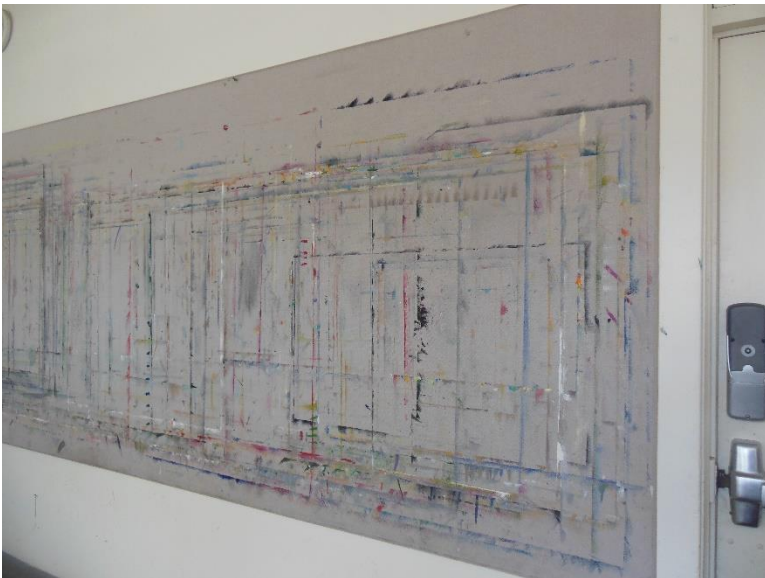
AI4. Classroom 22; fabric covered tackboard, paint damaged.
