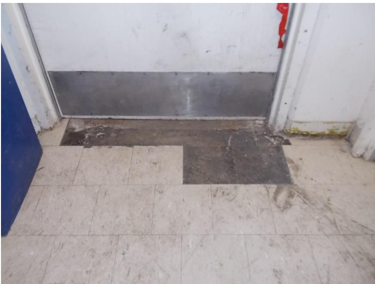
IF5. Basement; 9x9 VAT flooring damage.
