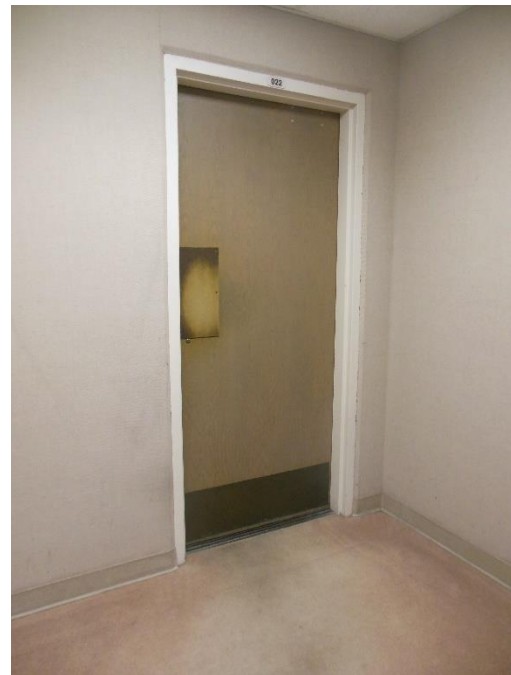
D4. Men's Restroom, 2nd floor; door and wall ADA signage not provided.
