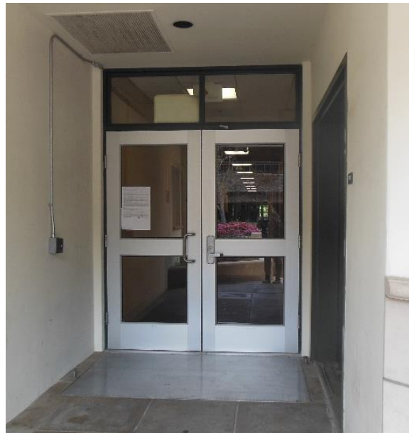
D4. Third floor entry; doors lacking wall mounted room ID signage.
