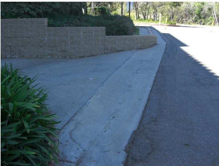
PT4. Non-compliant walkway at east main entry.
