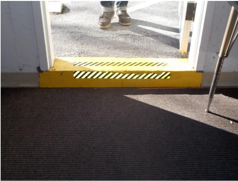
PT1. Room 32; door threshold exceeds 1/2" maximum.
