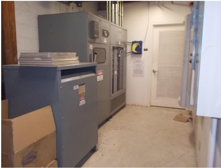
E1. Electrical switchgear.
