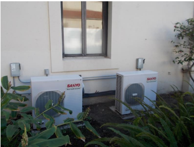
M4. Split heat pump systems for air conditioning offices.
