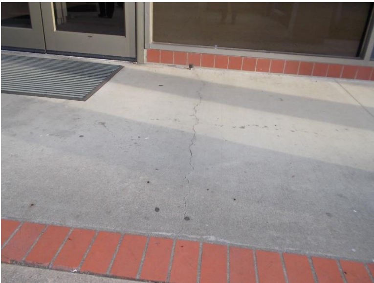
EF4. North side entrance; cracked concrete walkway.
