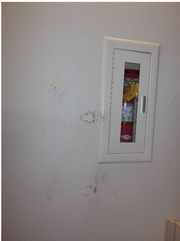
A7. Library lower level; wall damage.
