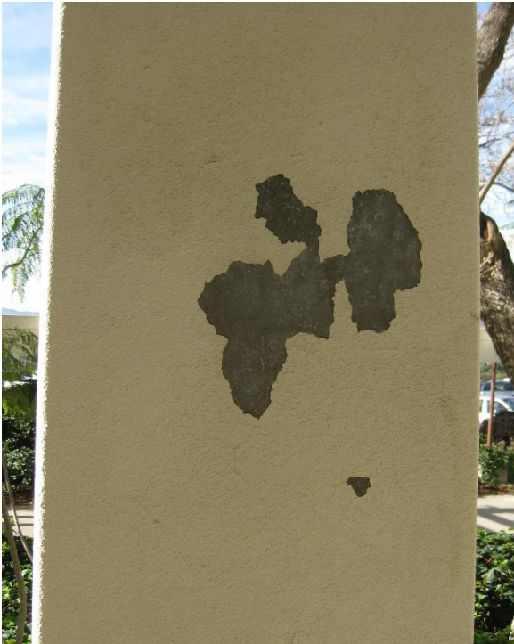
AE1. Exterior columns; peeling plaster paint.
