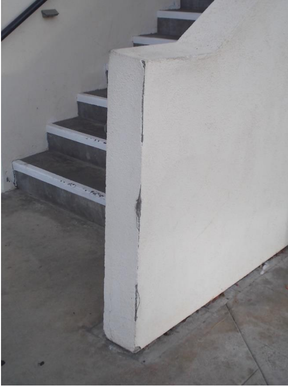
AE3. Exterior half wall; damaged plaster and paint.at corner condition.
