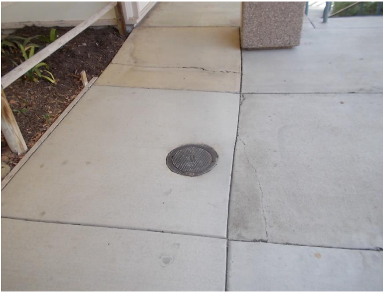
EF1. Exterior corridor walkway; cracked and degraded concrete.
