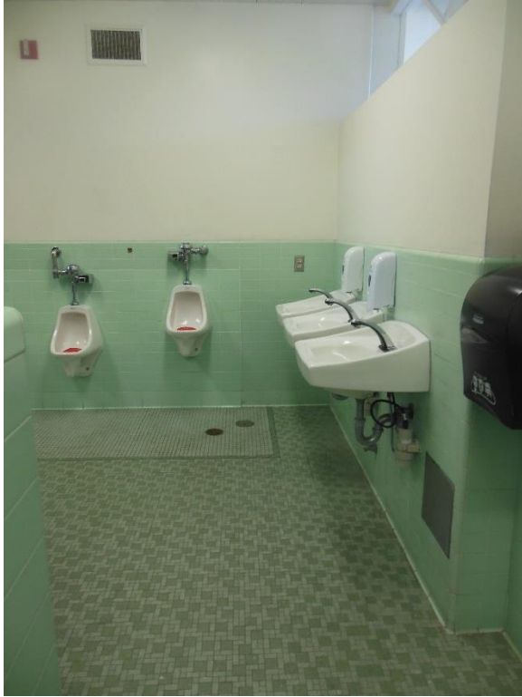
RR3. Men's Restroom; lavatories and urinals.
