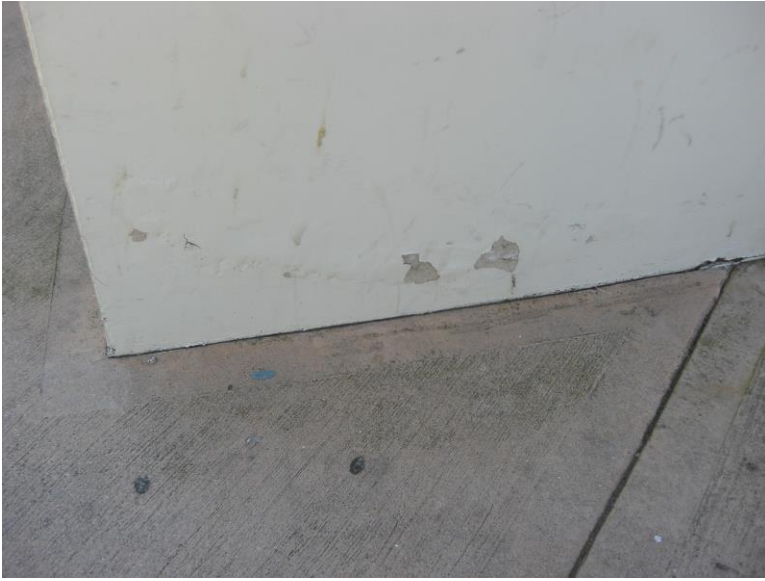
AE1. Exterior wall with paint damage.
