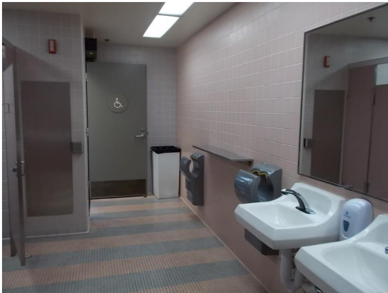
RR2. Womens restroom. Door signage does not meet minimum contrast requirements with adjacent surface.
