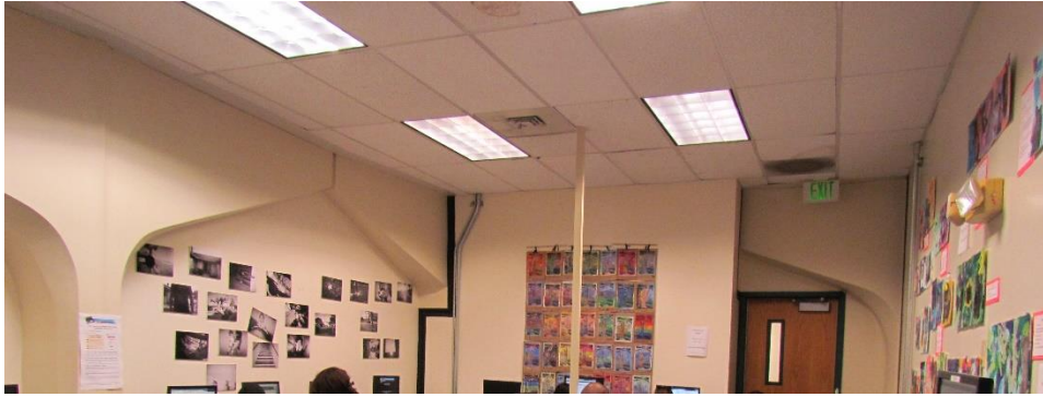
AI3. Second floor Atrium infill space; awkward wall transitions.
