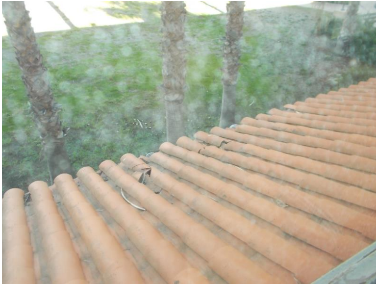
R1. Northeast roof overhang with damaged tiles.
