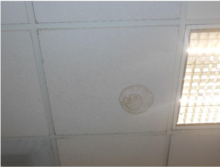
C1. Second floor classroom; stained ceiling tile.
