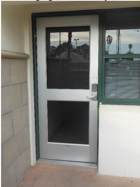
D3. Second floor entry Room 222; lacking wall mounted room ID signage, and pull-side clearance.
