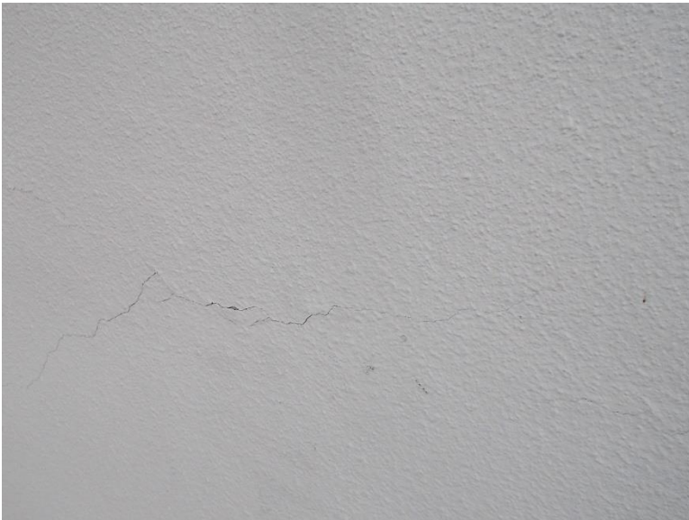
AE4. Exterior wall; cracked plaster finish.
