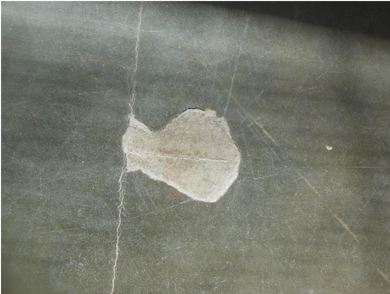
IF4. Classroom 22; concrete topping material damage.
