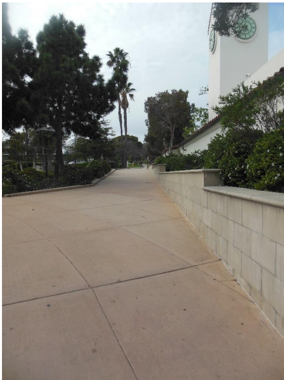
PT2. West side of building; excessive cross and longitudinal slopes along path of travel.
