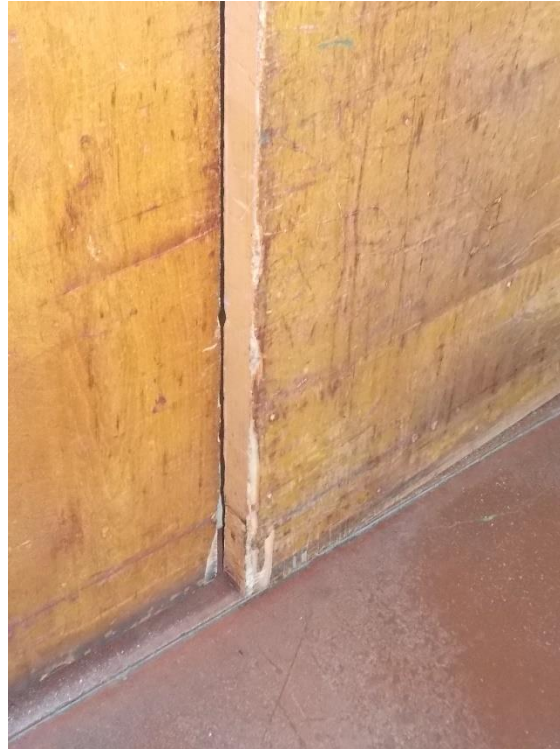
D2. Edge Damage at entrance doors.
