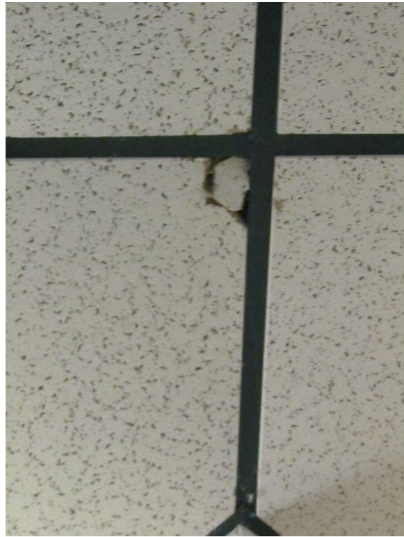
C2. Second floor; ceiling tile damaged.
