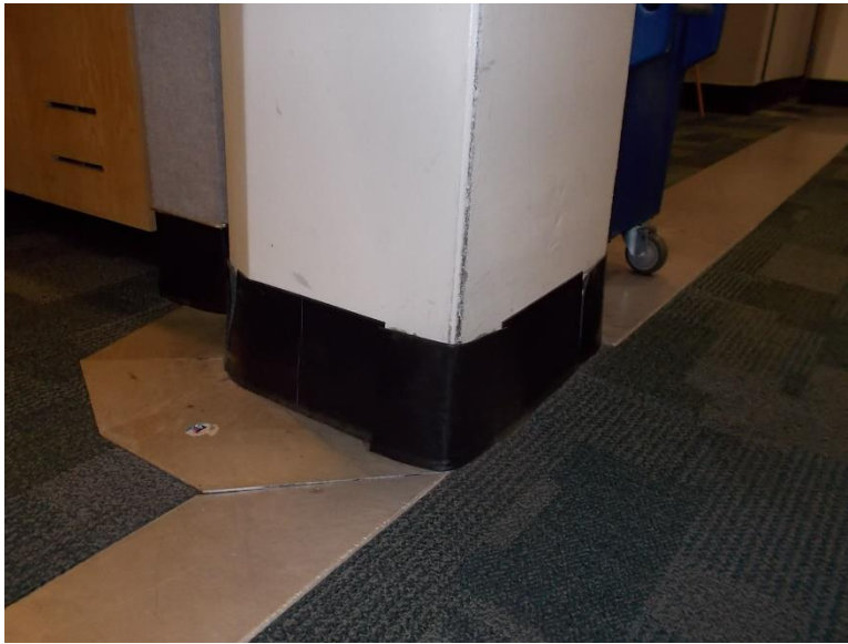
IF1. Second floor Atrium infill space; building expansion joint cover lifted, and rubber base damaged.
