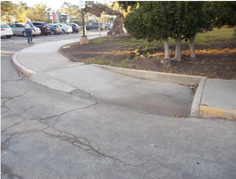
PT4. Non-compliant curb ramp at OE Auto Quad entry.
