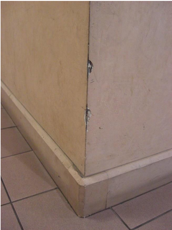
A2. Second floor corridor; veneer plaster corner damaged.
