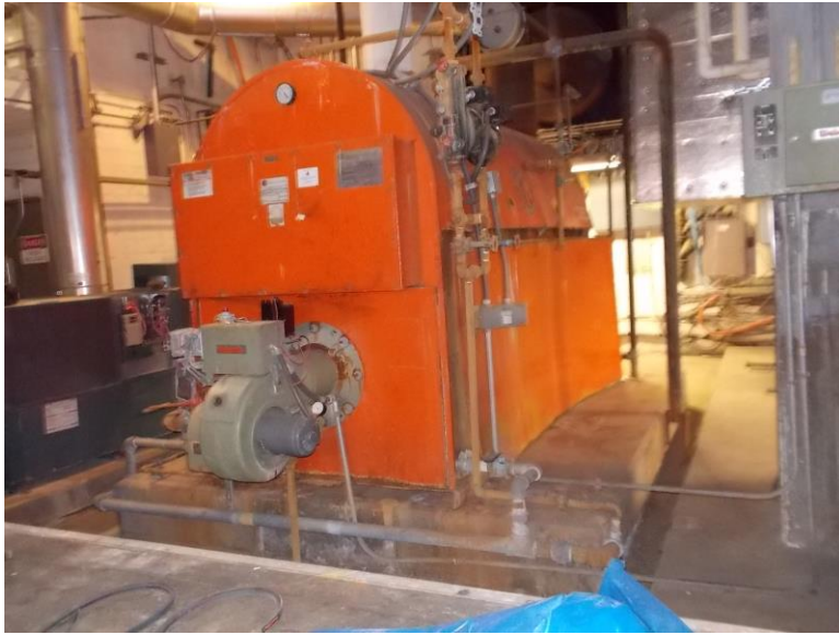
P1. Boiler in basement.
