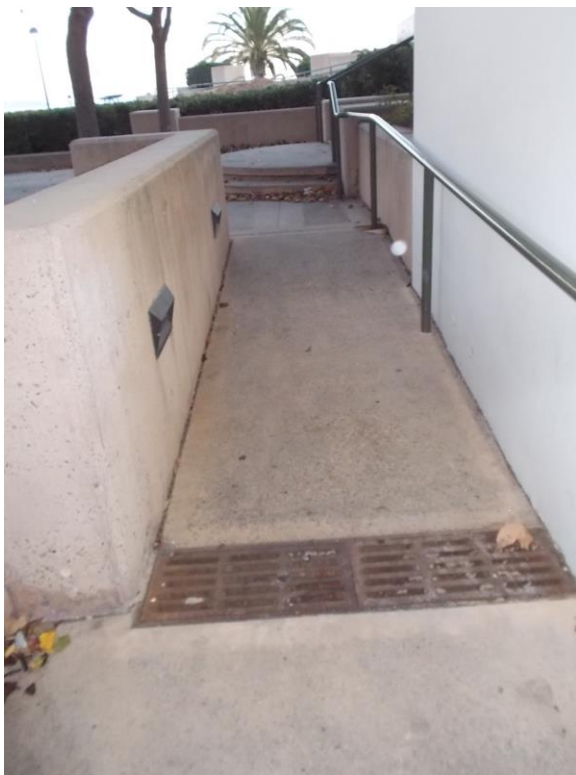
PT7. South side of building, ramp leading to Room 101; One handrail missing, non-compliant height at existing handrail, and drain grate creates abrupt and non-level lower landing.
