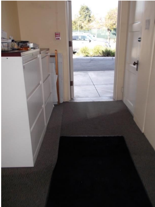
D1. Office 13; push-side clearance not provided, ramp is non-compliant, and adjacent door has non-compliant hardware and opens into the ramp.
