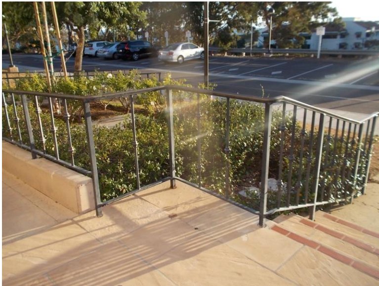
PT1. Non-compliant stairs at West main entry.
