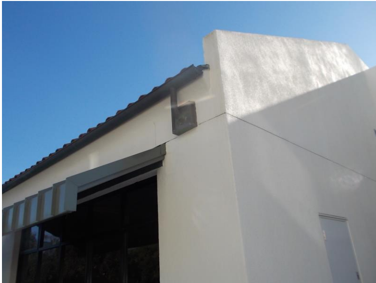
AE1. Exterior walls, minor plaster cracking.
