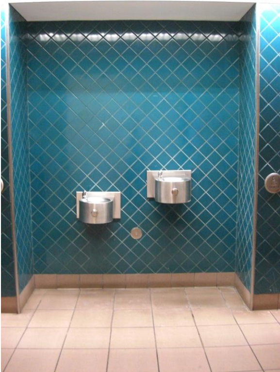
DF1. Second floor; hi-low drinking fountains.
