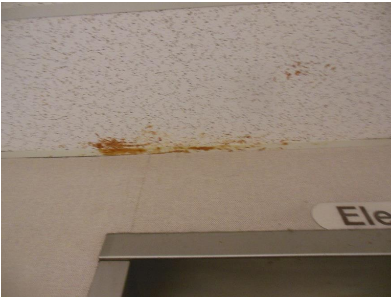
C4. Library upper floor; stained ceiling tiles at elevator.
