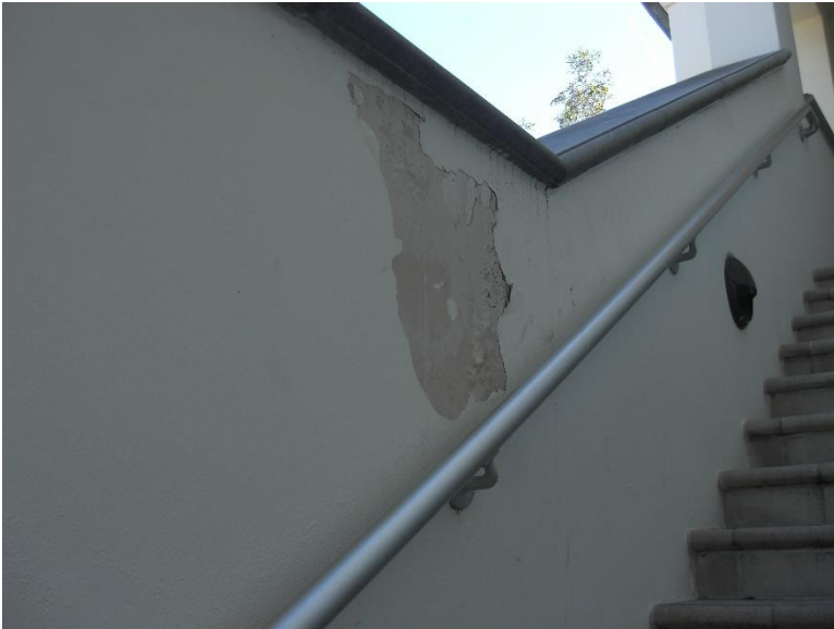
AE4. Exterior east staircase with peeling paint.
