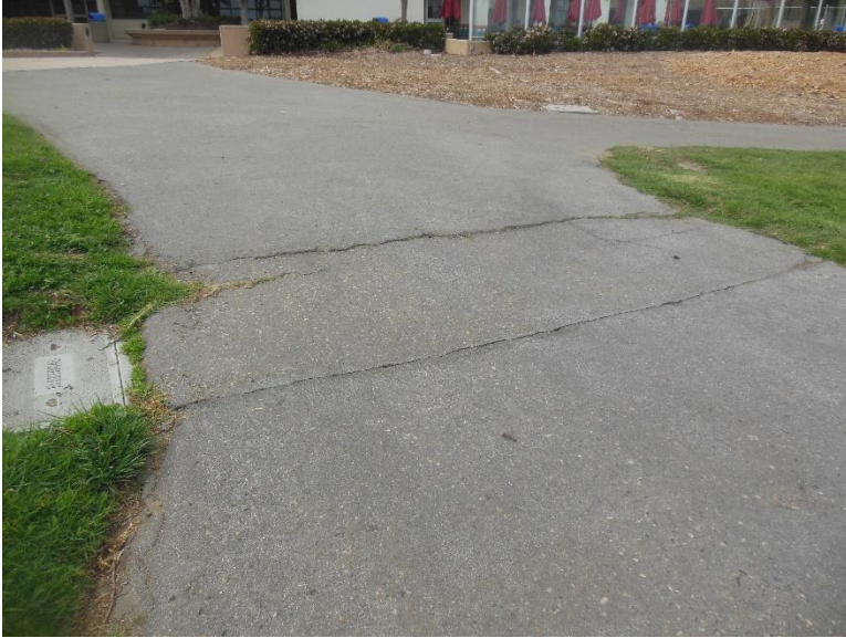
PT8. South side of building; excessive cross and longitudinal slopes, and abrupt change in level and hazardous surface features along path of travel.
