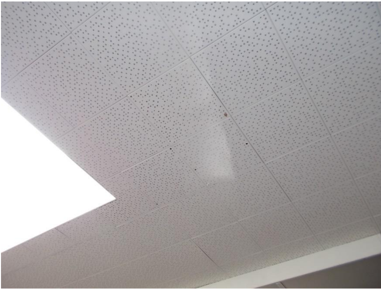
C1. Classroom; glue on ceiling tiles, typical.
