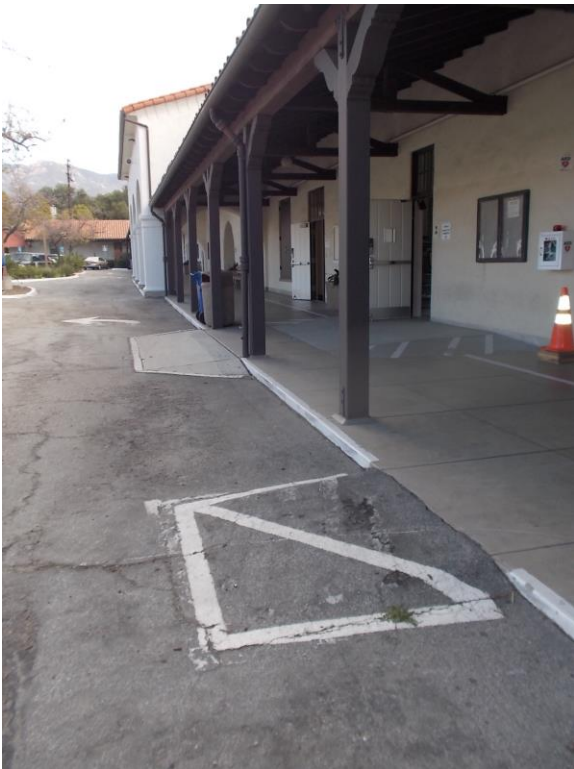
PT4. Curb ramps to parking lot; ramp cannot project into the path of cars, and are missing truncated domes. Asphalt surface is degraded.
