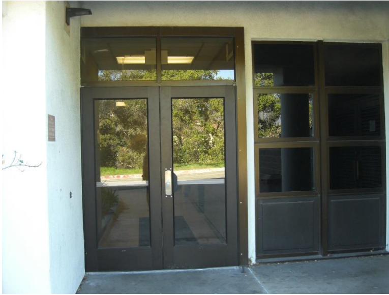
D1. First floor south entrance doors. Doors are lacking code required signage and ISA symbols.
