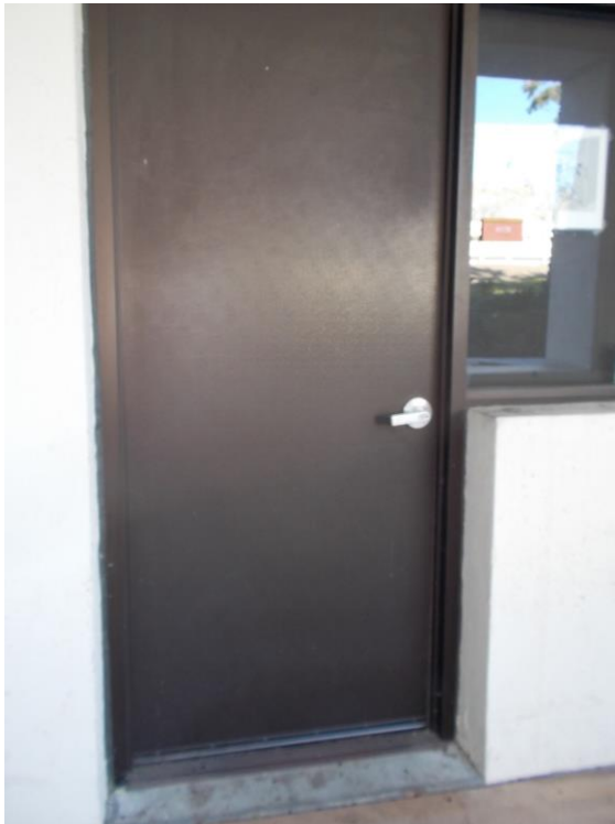
D3. Painted office door at north east side of building, with non-compliant threshold.
