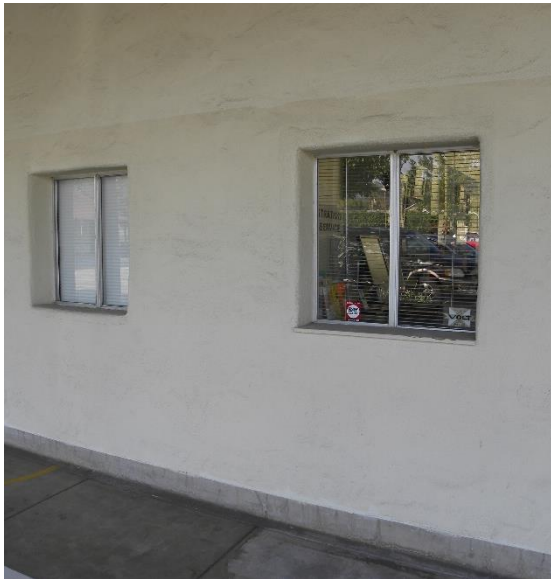
EW3. Exterior aluminum windows; frames don't match other existing windows.
