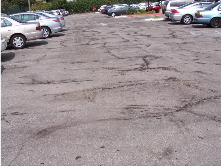
EF3. Asphalt parking lot; degraded materials, poor condition.
