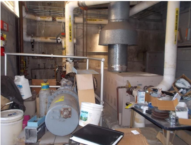
M2. Mechanical equipment blocked by debris.
