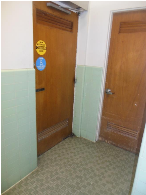
RR5. Mens foyer; door clearances not provided.
