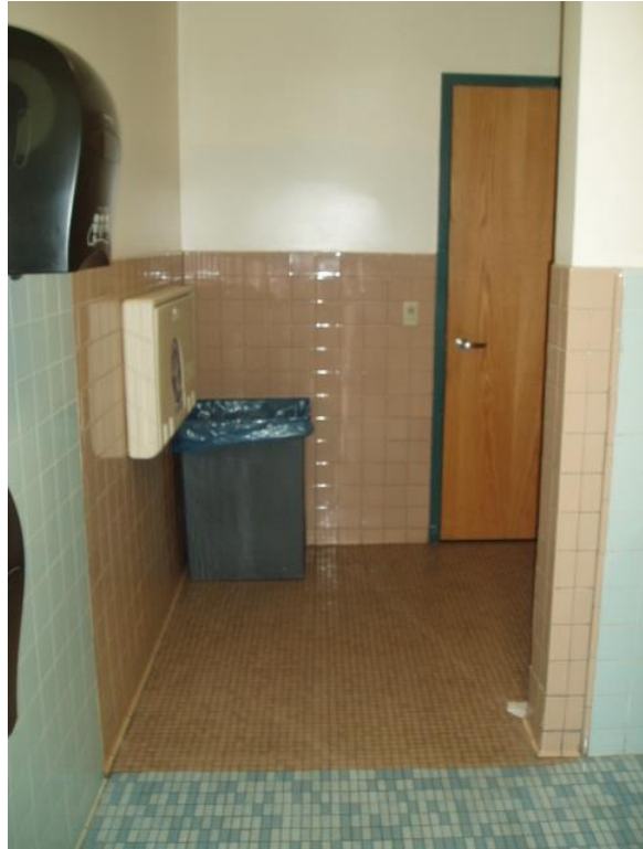
A16. Restroom wall tile mismatched.
