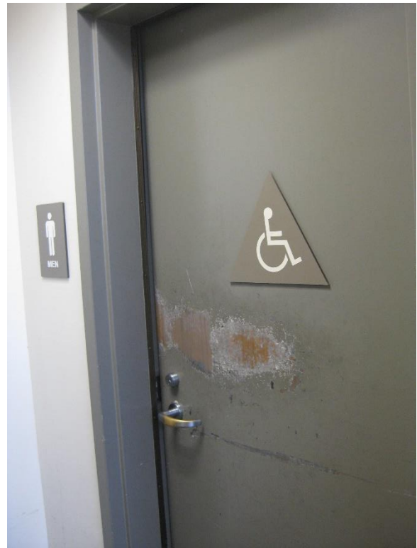
D2. Lobby Men's Restroom; damaged paint, and non-compliant door signage.
