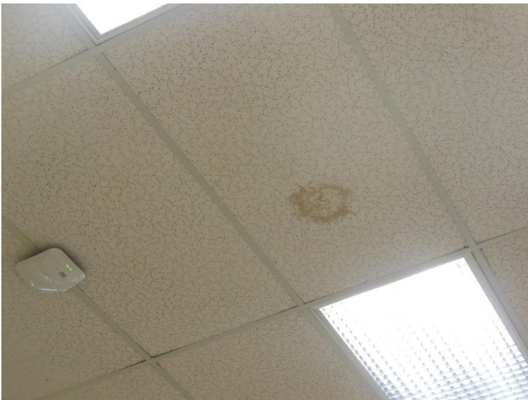
C2. Library second floor; stained ceiling tile.
