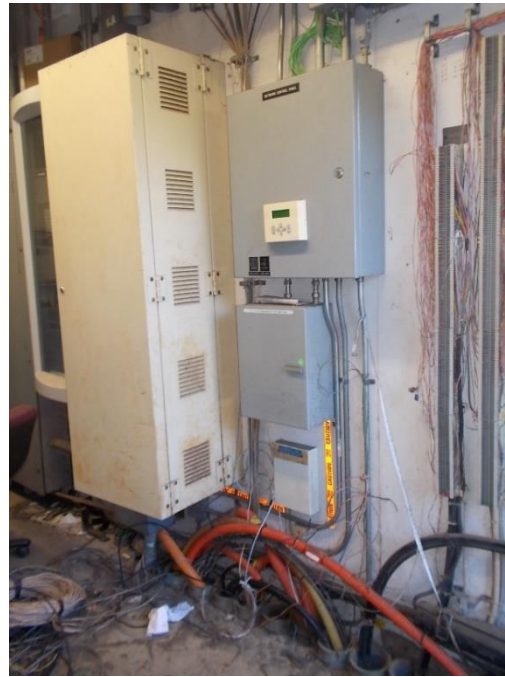
E2. IT and Fire Alarm equipment.
