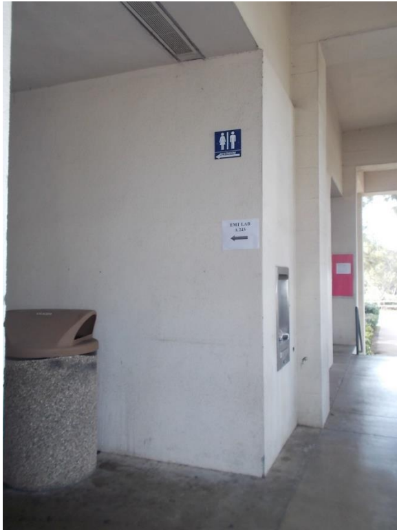
S5. Non-compliant RR signage – 2nd floor.
