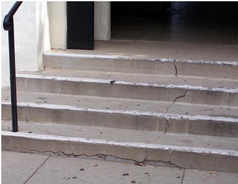
ST2. Stairs at west entrance; non-compliant handrails, stair nosing faded, and degraded concrete materials.
