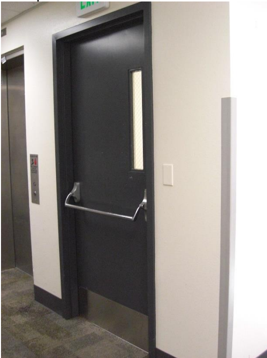
D2. Third floor stairwell door; crossbar style panic hardware does not match other exit doors touchpad style.
