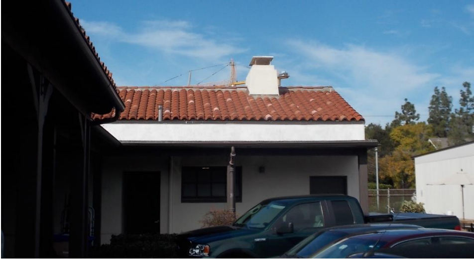
R3. Kitchen; clay tile and roof chimney/vent, and built-up roofing over walkway canopy.
