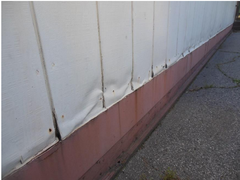
AE4. Portable building, exterior painted siding, damaged.
