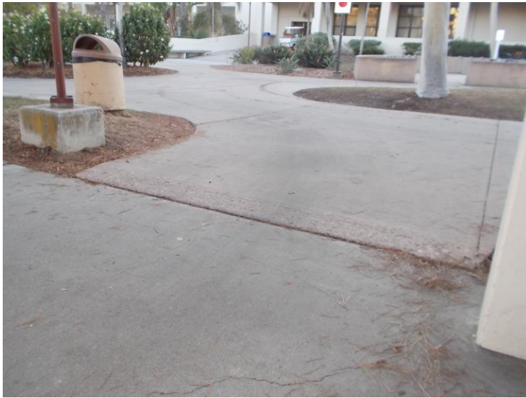
EF1. Exterior walkway; abrupt changes in level.
