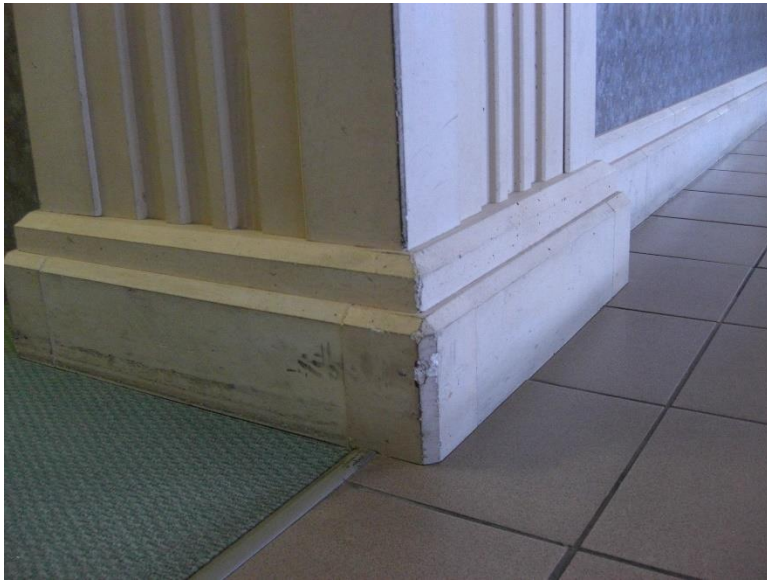
IF1. Second floor reception; wood base damage.
