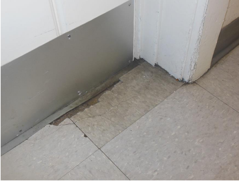
IF1. Main Office Room 8, damaged VCT at door.
