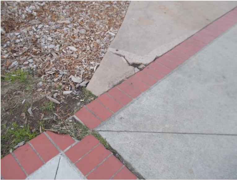
PT3. Non-compliant transition at East ramped entry.
