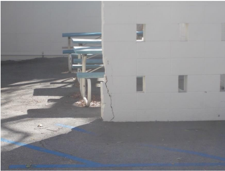
AE1. Exterior patio CMU wall; damaged.
