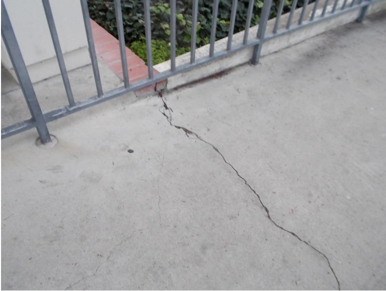
EF3. Northeast exterior walkway at top of ramp; cracked concrete.
