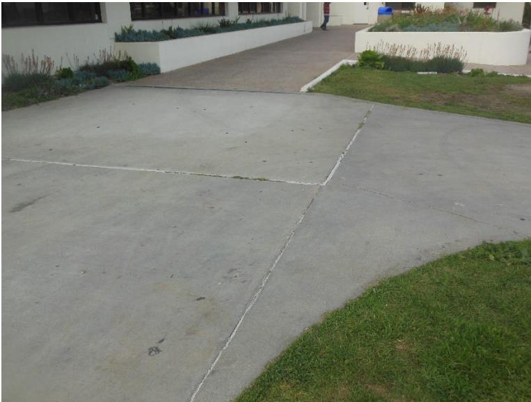
EF2. South side concrete walkway, with excessive longitudinal slope and deteriorated expansion joints.
