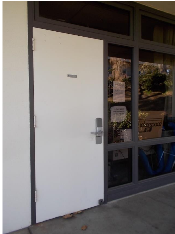
D4. Classroom door at OE build first floor storefront system.
