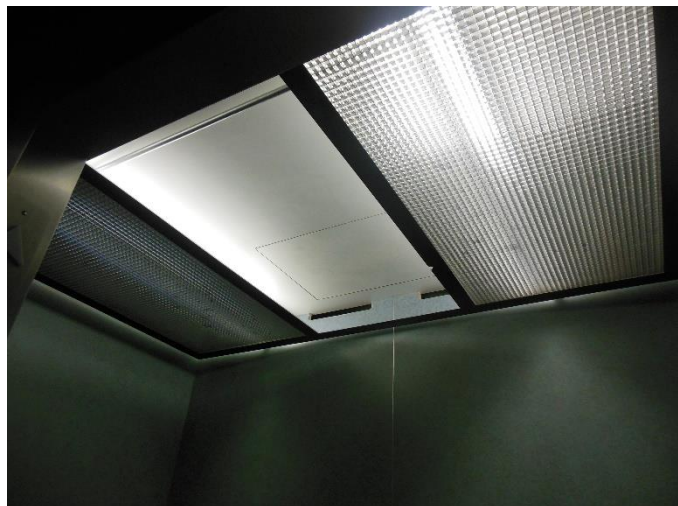
EV4. Elevator car ceiling; missing light lens.
