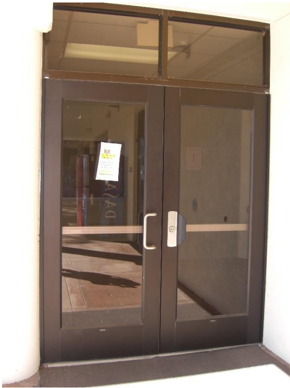
D3. First floor west lower entrance doors; Right hand door abuts the adjacent wall without providing hand clearance to avoid pinching.
