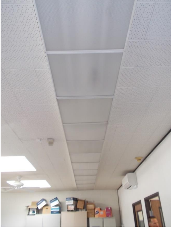
C3. Office 2; glue on ceiling tiles with surface mounted lights.
