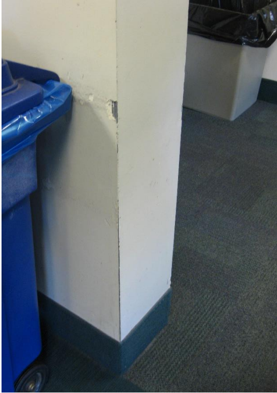
A15. Wing wall damaged corner.
