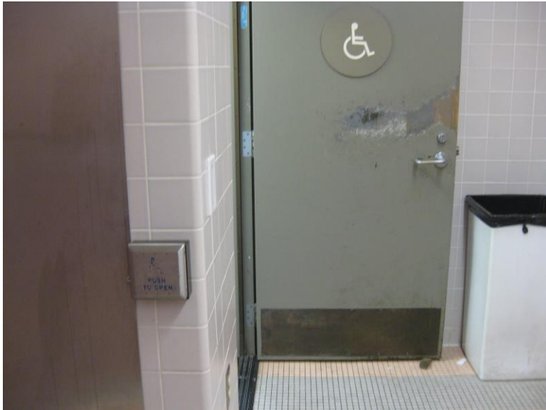
RR1. Women's Lobby restroom. Door finish repair required. Low level access button for electronic door operator is required by code, and ADA door signage is non-compliant.
