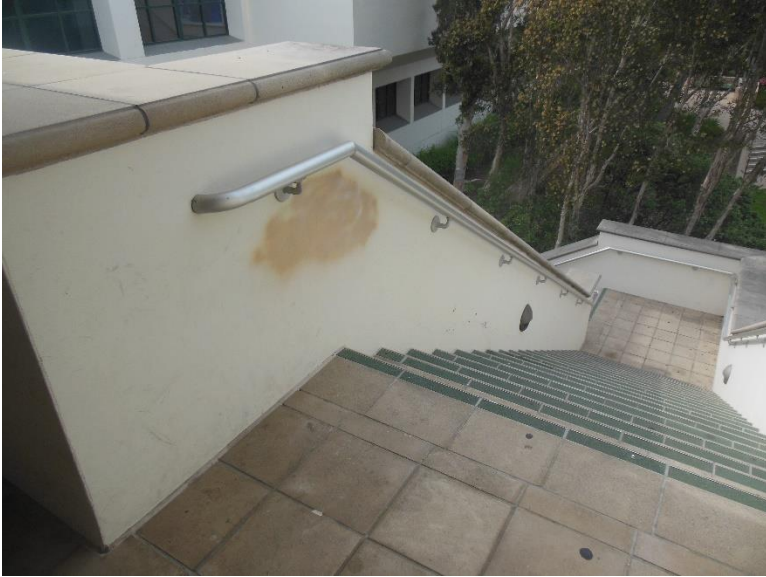
AE3. Exterior east staircase with paint damage.
