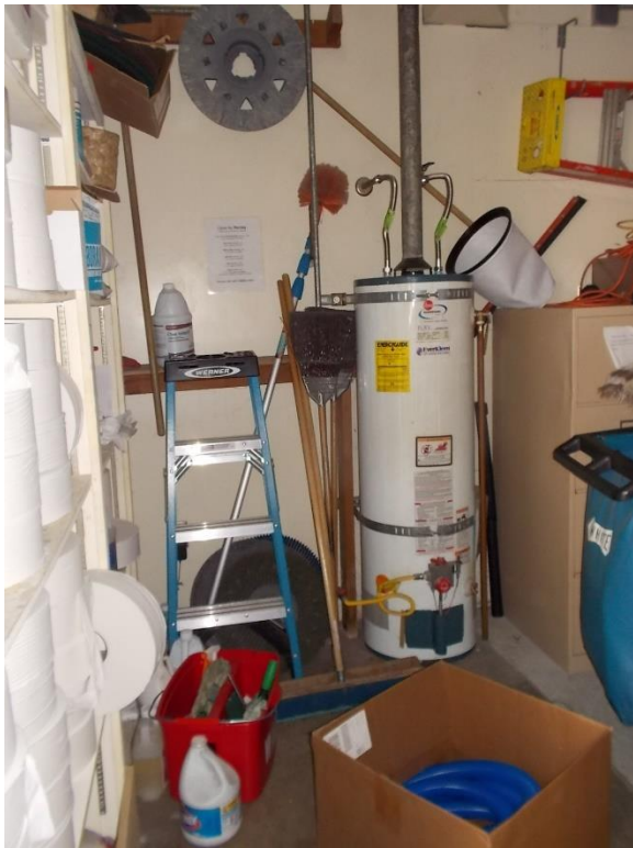
M5. Hot water heater, clear floor space not provided.
