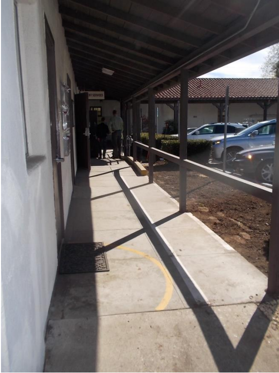
PT7. Exterior walkway; path of travel interrupted door swing, and curb edge not provided.
