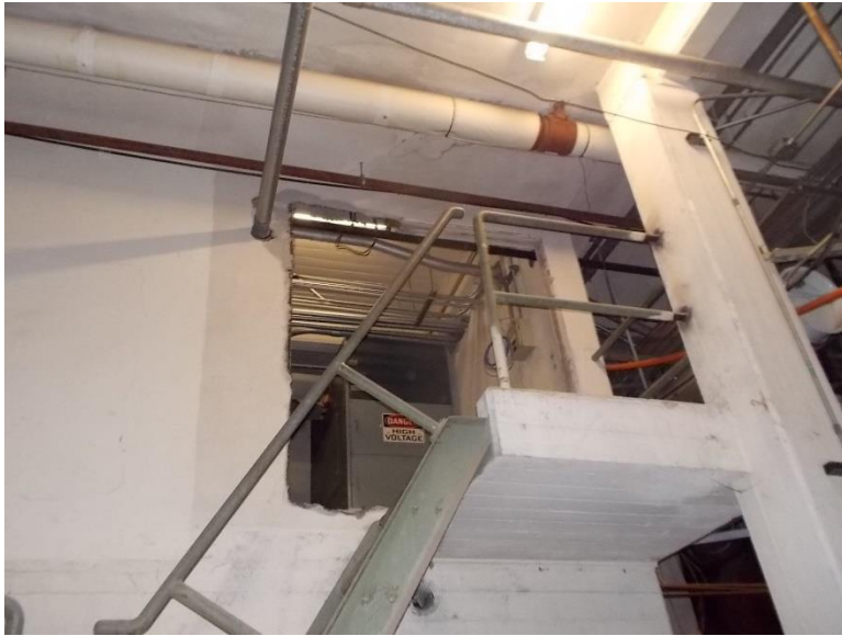
E3. Access to Electrical equipment in basement.
