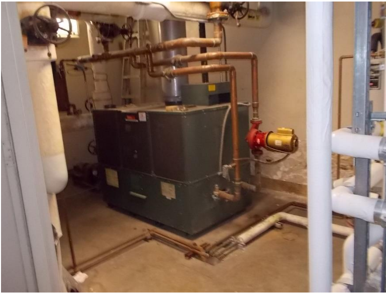
M1. Boiler in basement.
