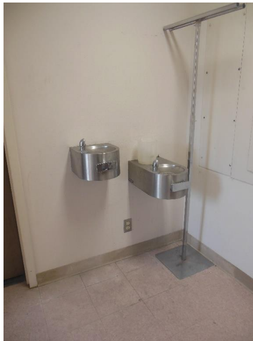
DF5. Top of Stairwell 136; non-compliant hi-low drinking fountains.
