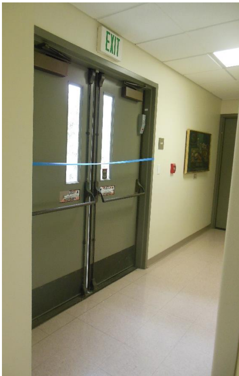
D6. Exit doors, Corridor 112A; exit access blocked with tape.
