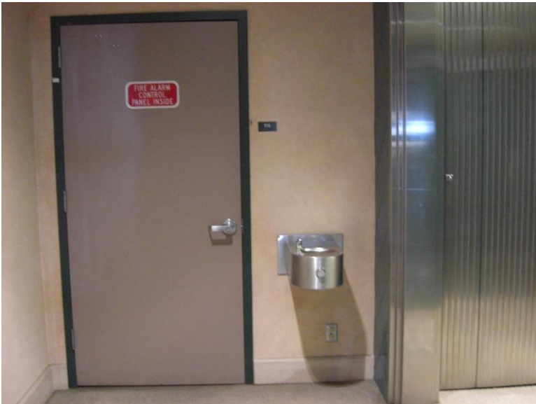
DF3. First floor single drinking fountain; maneuvering clearances not provided.
