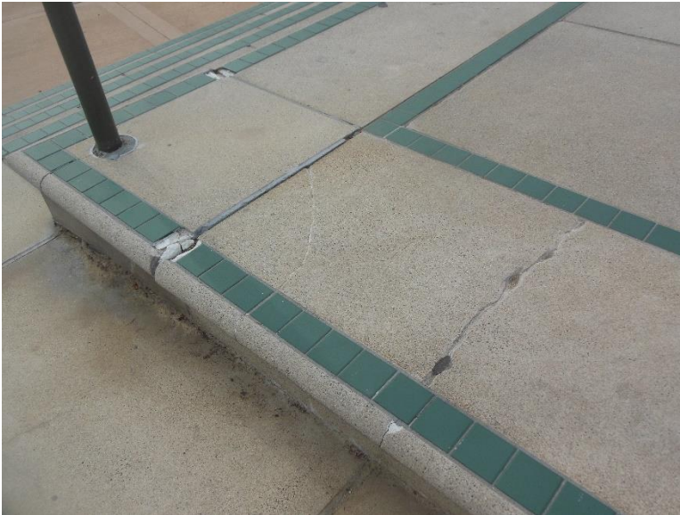
EF2. Front entry plaza stairs; concrete cracks and tile missing.
