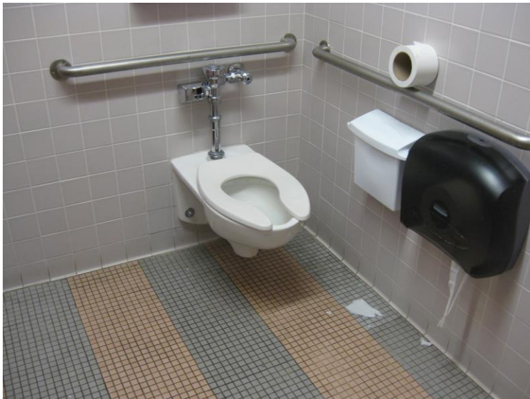
RR2. Women's Lobby Restroom. Dispenser and disposal units protrude into required clear space below handrail.
