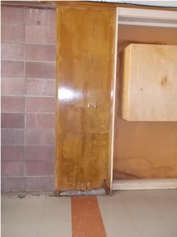
AI1. Auditorium; water damaged exposed CMU and wood finishes.
