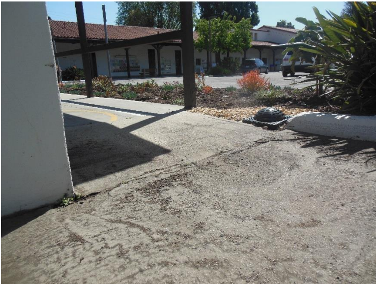
PT8. Exterior walkway; path of travel with hazardous surface feature and no level landing at bottom of ramp.
