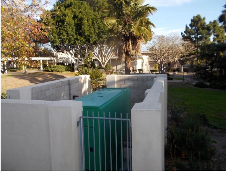
E1. 2006 New generator behind east side of the building.
