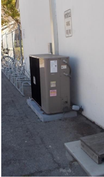
M1. Outside Room 1; mini-split heat pump system.
