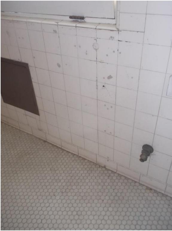
AI1. Women's Restroom, ceramic wall tile damaged.
