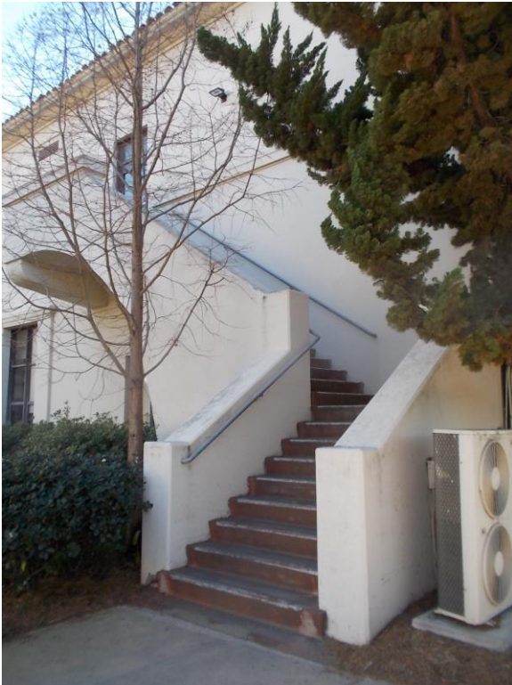
S4. Exterior stairs with non-compliant handrails, and no level landing.
