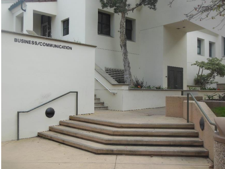
PT6. East side of building; non-accessible entry lacks wayfinding signs directing user to ramped entry location.
