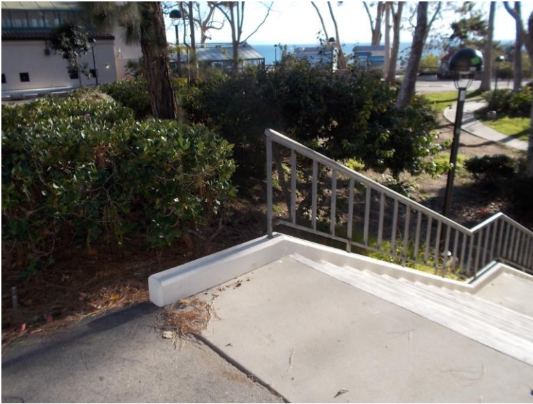
S3. Exterior stairs to OE with non-compliant handrails.
