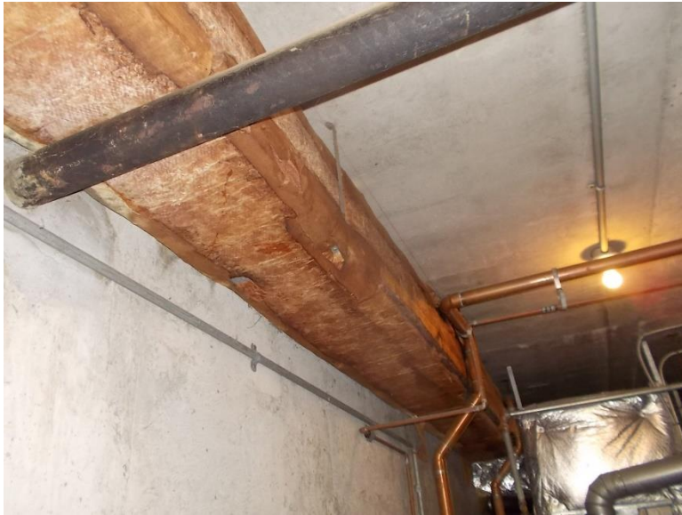
M4. Mechanical space under Kitchen; exposed insulation.
