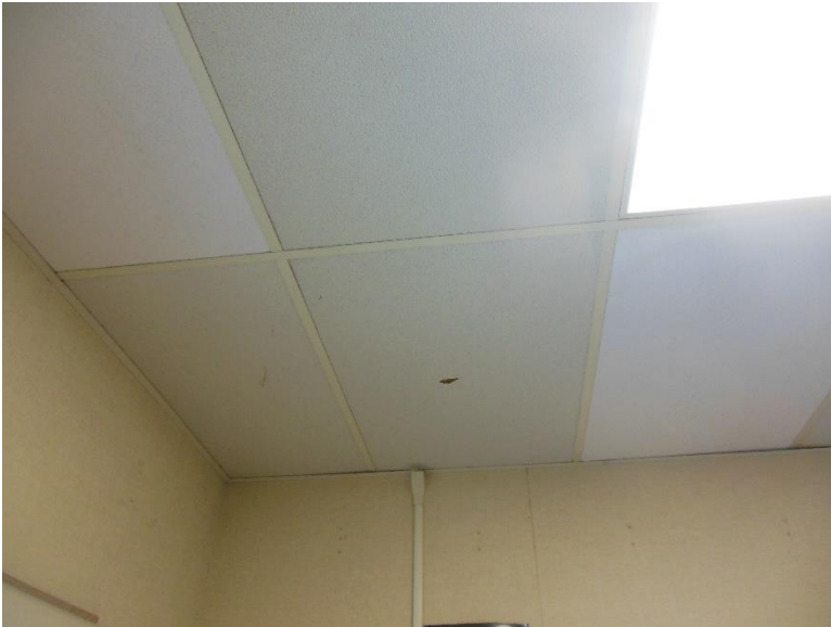
C4. Portable Classroom 29; damaged and miss-matched suspended ceiling tiles.
