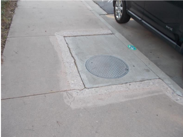
PT3. Exterior sidewalk; non-compliant path of travel. Abrupt changes in level.
