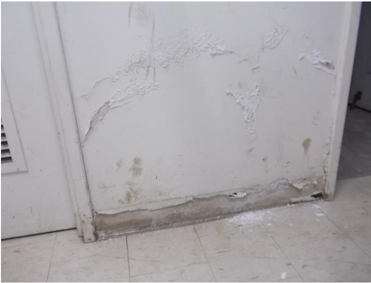
AI1. Basement; interior drywall and base damage.
