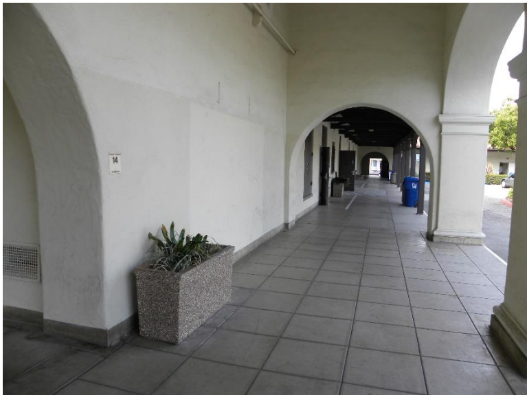
AE2. Permanent building exterior wall; painted plaster, non-matching colors.
