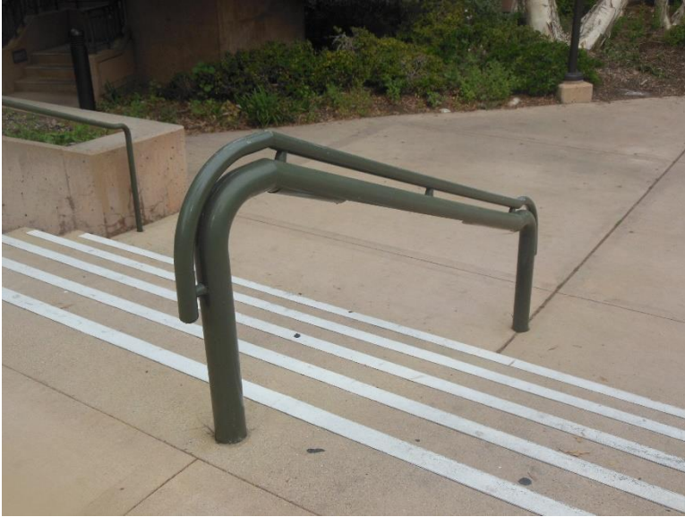
ST7. North side of building; exterior stair with non-compliant handrail heights and returns.
