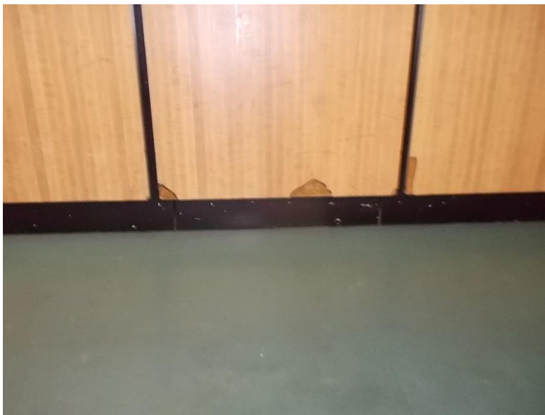
AI4. Elevator cab interior; damaged wall panels.
