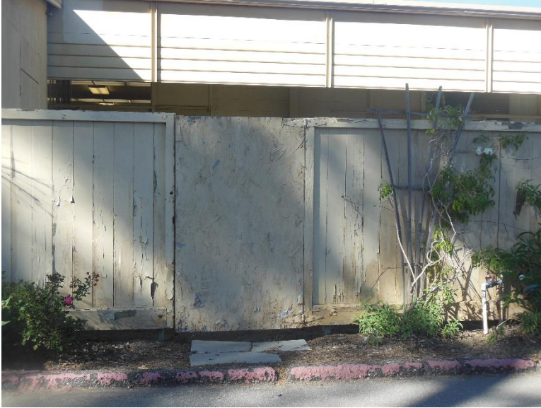
AE3. Exterior wood patio fence; damaged paint.
