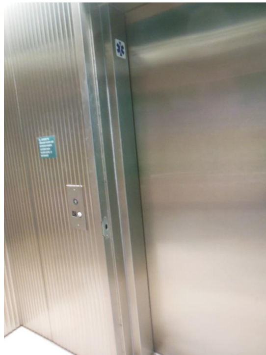
EV2. Braille floor level signs lacking.
