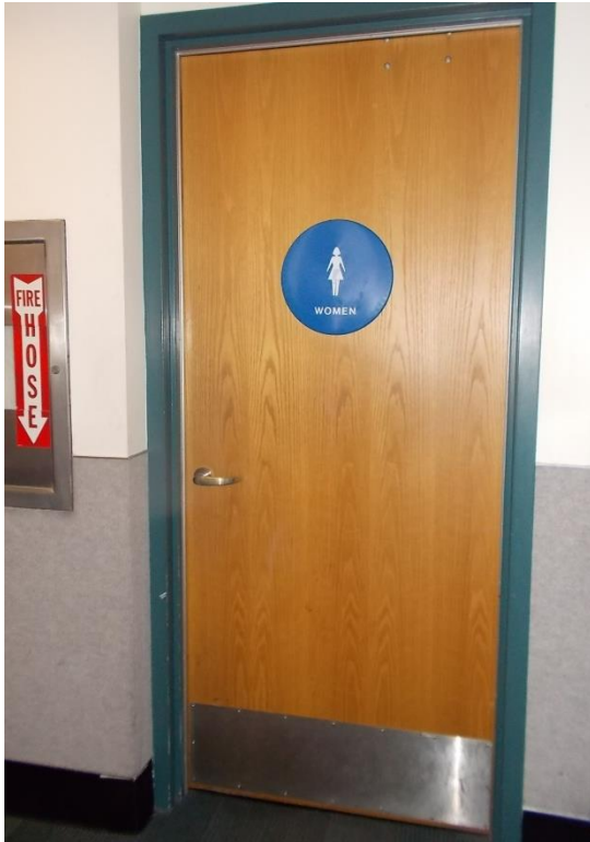
S1. Women's Restroom entrance; wall mounted room ID sign missing.
