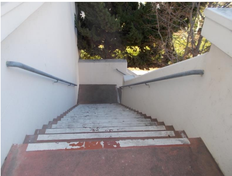
S2. Exterior stairs with non-compliant nosings and handrails.
