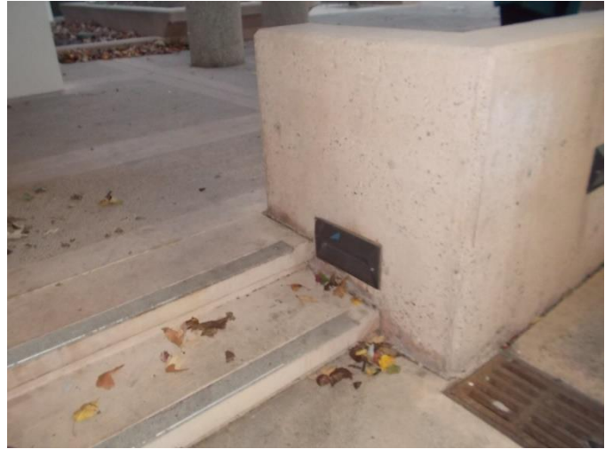
ST2. Exterior south stairs; missing required handrails.
