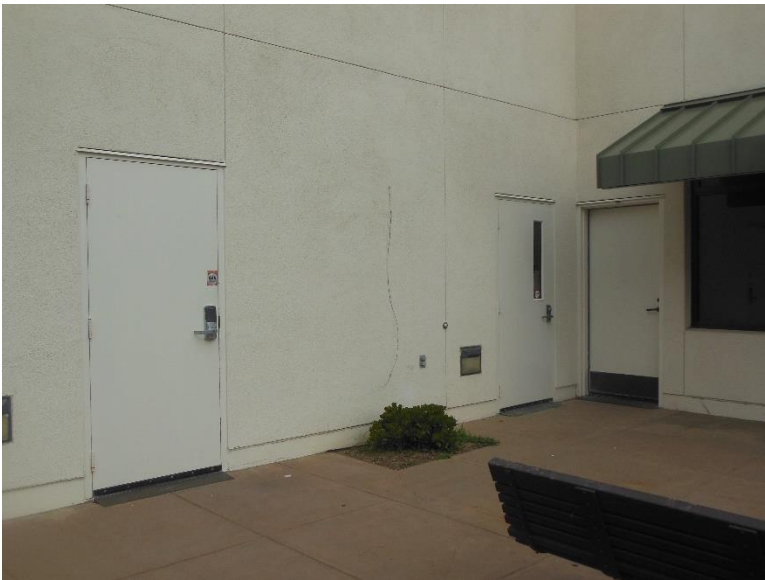
D4. Doors on east side of building; lacking code required wall mounted door identification signage.
