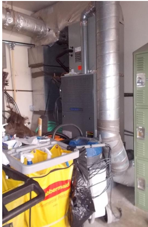
M2. Gas fired forced air heating units; clear floor space not provided.
