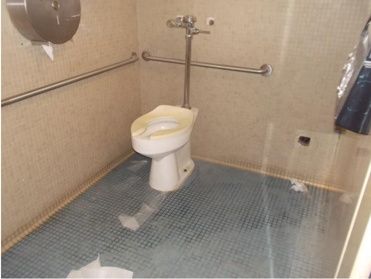
RR3. Men's Restroom accessible stall; ceramic wall finishes have holes and dispenser mounting location interferes with the required clear space above side handrail.
