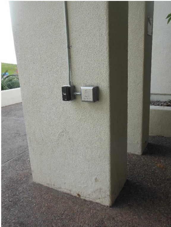
D2. Main Entrance; low level access button for electronic door operator not provided.
