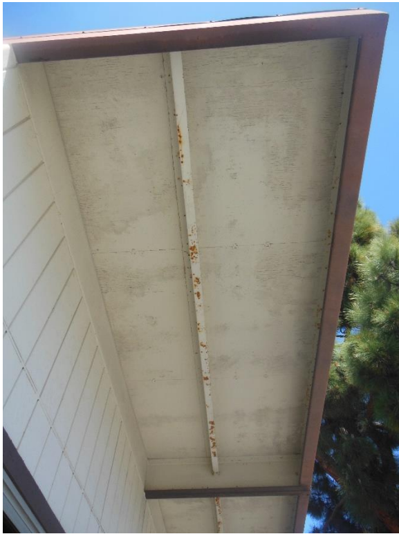
R1. Portable Classroom 28A; underside of roof overhang, rusted.
