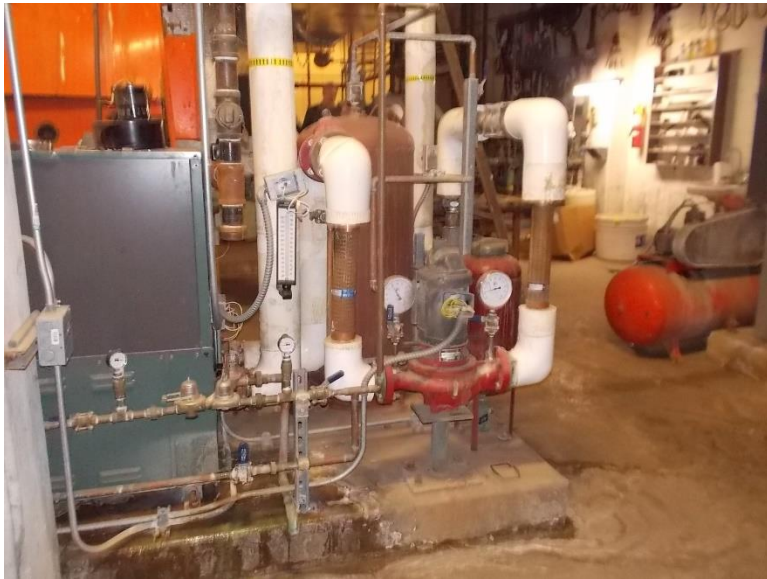
P2. Boiler piping in basement.
