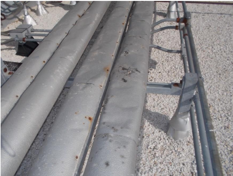
M2. Rooftop mechanical piping damaged.
