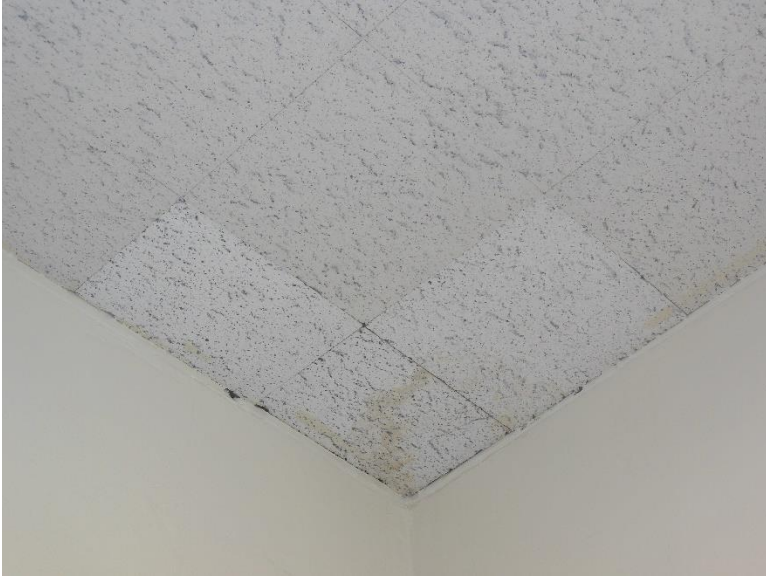
C3. Copy Room 10; glued on ceiling tile, damaged.
