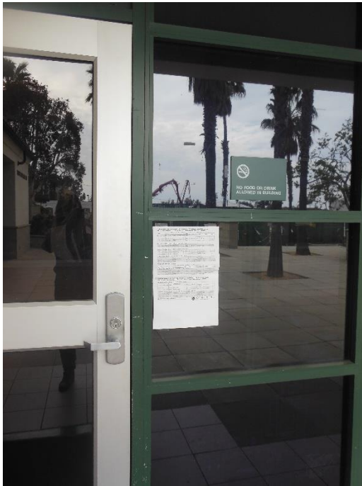
D1. Main entry; lacking wall mounted room ID signage, and an ISA symbol.
