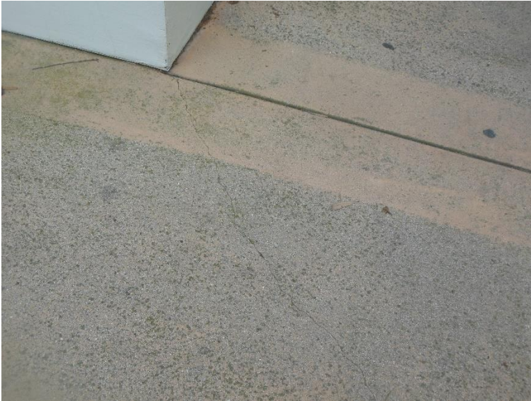
EF1. Colored concrete walkway with cracks.
