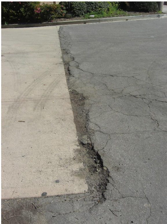
PT2. Asphalt to concrete transition along path of travel from the IDC building to the parking lot is crumbled, uneven and degraded.
