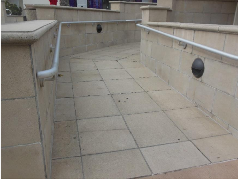
PT3. West side ramp to main building entry; intermediate landing exceeds the 2% allowed maximum cross slope.
