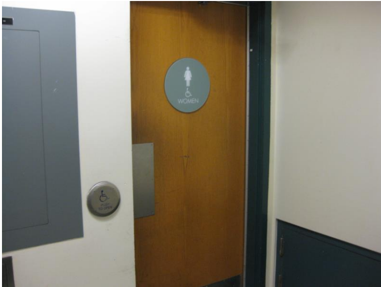
RR1. Women's Restroom; wall mounted ADA signage and electronic door opener lower-level push plate not provided.
