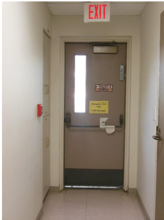
D7. Exit door, Corridor 008, push-side clearance not provided.
