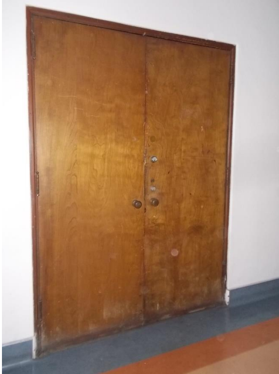
D1. Second floor equipment room doors.
