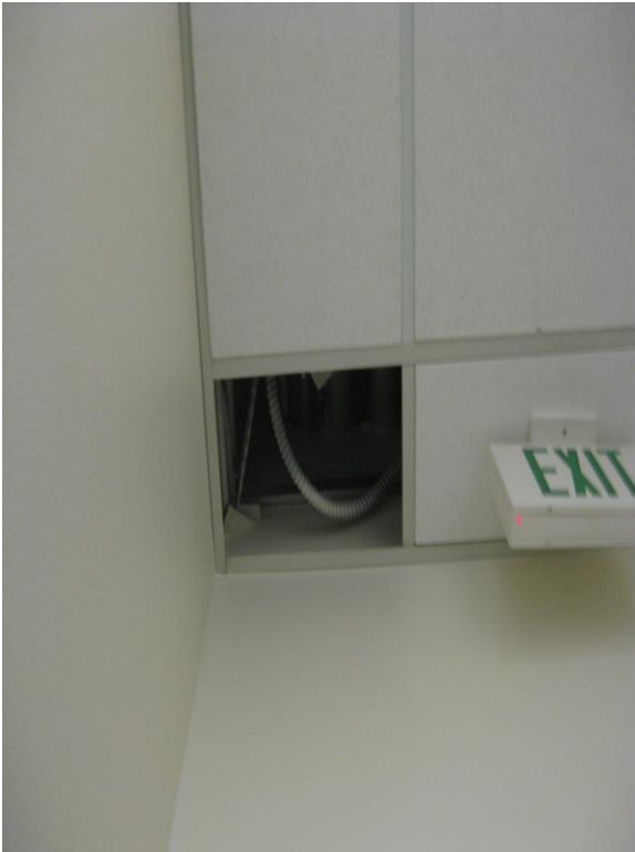
C1. Corridor 112B; missing ceiling tile.
