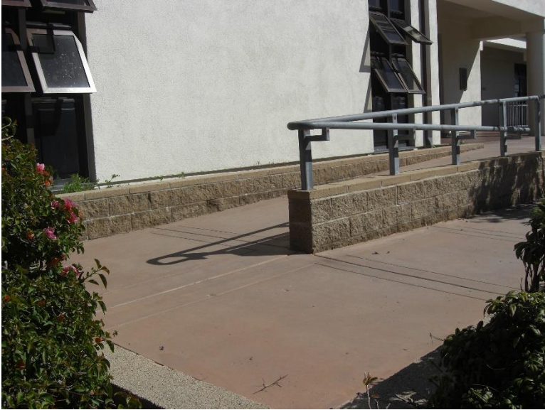
PT3. Non-compliant ramp at west main entry.
