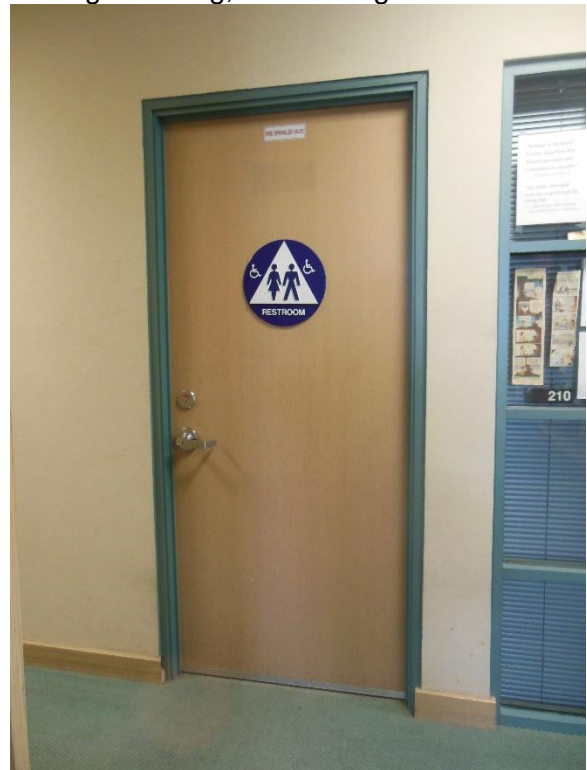
D7. Second floor staff unisex restroom. Missing wall mounted room ID signage.
