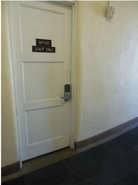
D3. Office 15; interior painted wood door, ADA room ID signage not provided.
