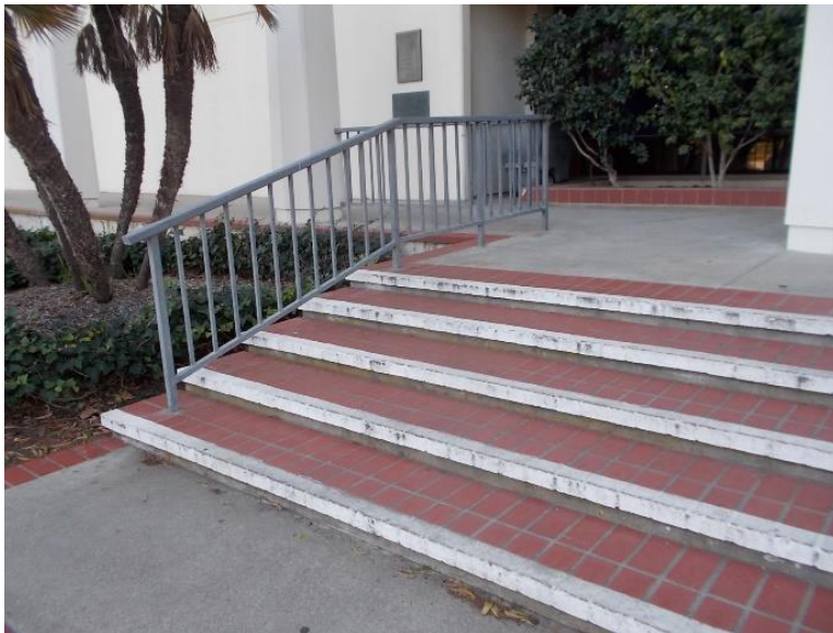
S2. Exterior east stairs; lower handrail extensions are non-existent, gripping surface is too wide, the top and bottom landings have excessive slope and are not level.
