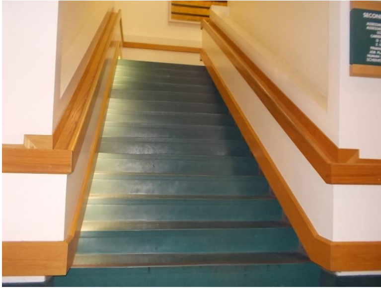
S3. Interior staircase; stair nosings not contrasting, handrails not compliant, and stair signage not provided.
