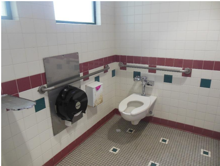
RR4. Cafe restrooms; dispensers may impede forward clear space at accessible stall.
