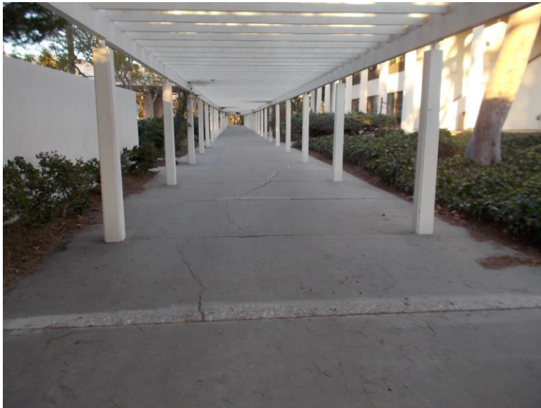
EF2. Exterior walkway; cracked concrete, excessive slopes, and abrupt changes in level. End of walkway terminates into fire truck lane.
