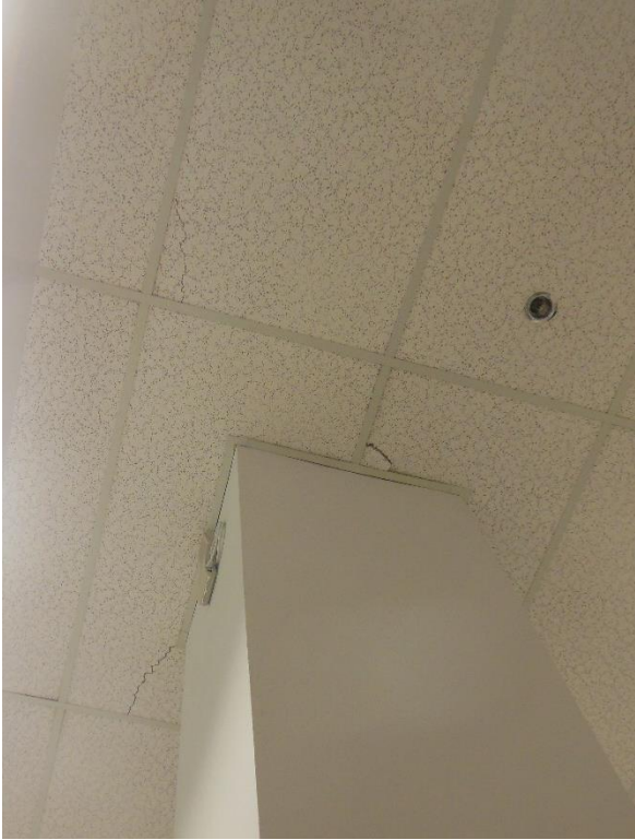
C3. Library upper floor; broken/damaged ceiling tiles.
