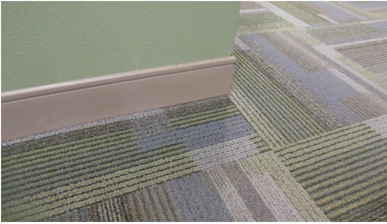
IF1. Learning Center carpet tile and wood base in excellent condition.
