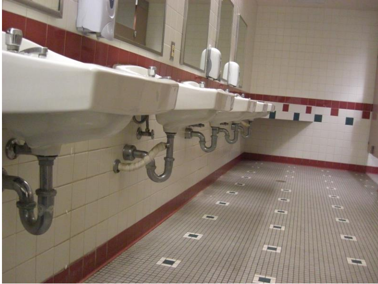
RR3. Second floor restrooms; knee protection is not provided at under sink plumbing trap.
