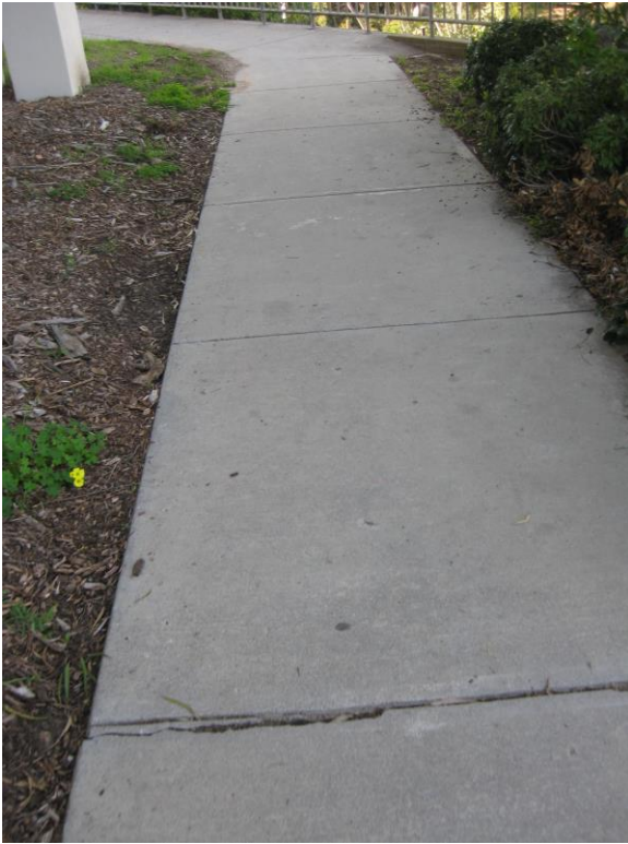
EF1. East side concrete walkway, with large cracks, tripping hazards and excessive cross slope.
