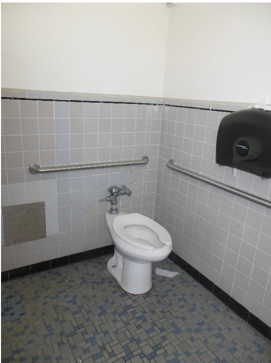
RR4. Men's Restroom; toilet paper dispenser located too high above toilet, and protrudes into clear space above grab bar.
