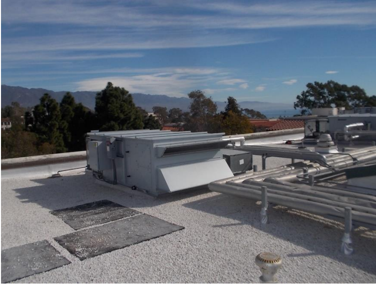
M1. Rooftop mechanical equipment.
