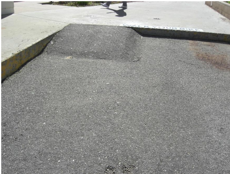
PT4. North side of building; non-compliant asphalt ramp.
