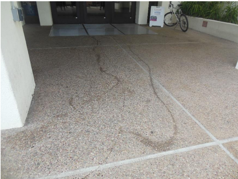
EF4. Main south entrance walkway; stained pebbled finish surface.
