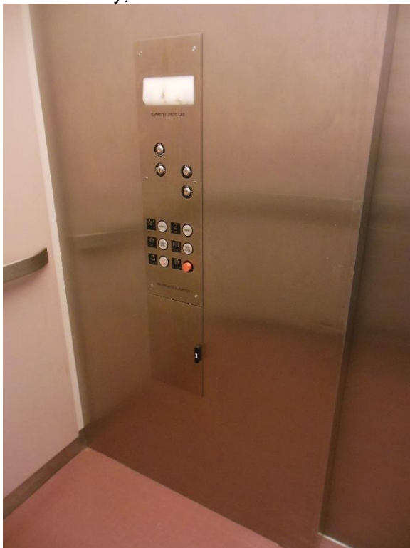
EV2. Elevator interior cab controls.
