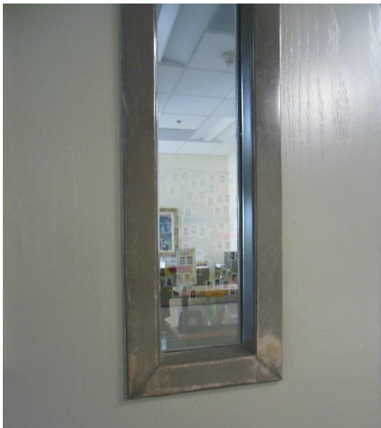
D3. Office 121; damaged frame at door lite.
