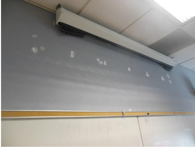
A5. Second floor classroom; wall repair damage.
