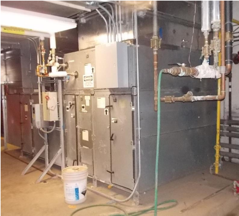
M2. AHU in basement.
