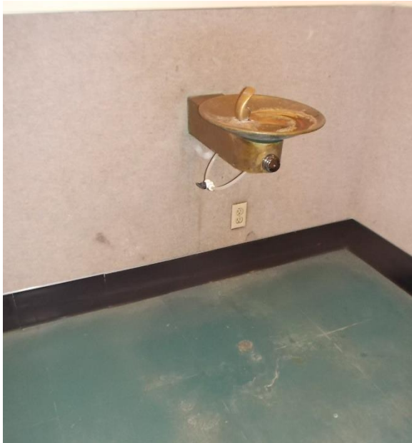
DF1. First floor single drinking fountain; hi-low drinking fountain not provided and flooring damaged.
