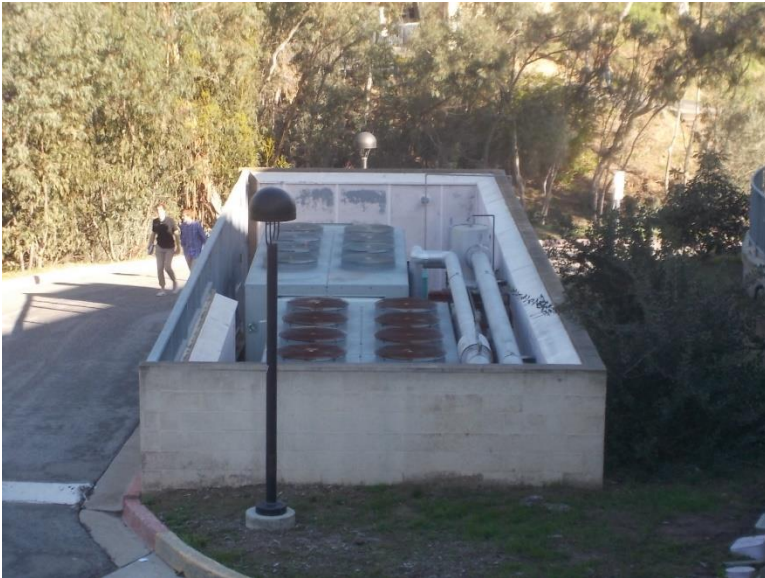
M1. Chiller enclosure. One unit is in use and in good condition.
