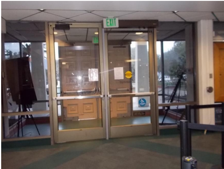
D1. First floor north east exit; electronic door operator low level access button required by code is not installed, and tactile exit signage not provided.
