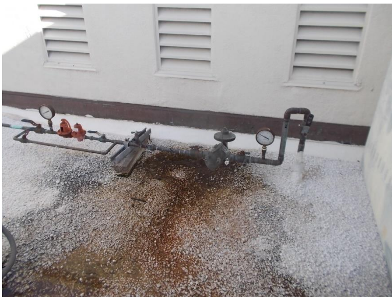
R2. Mechanical roof well with water damage at built up roofing system.
