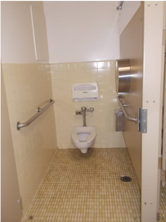
RR4. Women's Restroom ambulatory stall; wall finishes have holes and dispenser mounting location interferes with the required clear space above side handrail.
