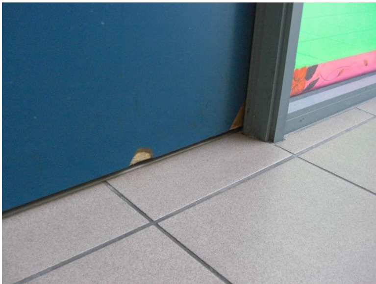
D3. Third floor; damaged and stained plastic laminate faced office door.
