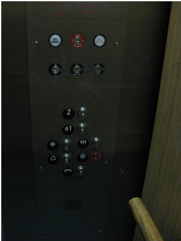
EV2. Elevator car interior.
