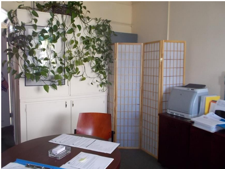
E2. Office 13 interior; main distribution panel, service meter, distribution panel and transformer, behind screen.
