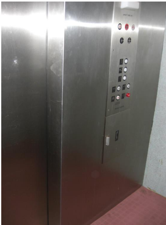
EV3. Elevator car interior.
