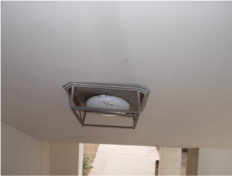
E5. Exterior lighting at northeast stairs.
