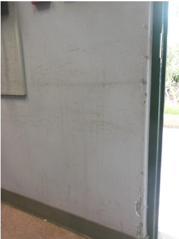
A7. Second floor classroom; wall and paint damage.
