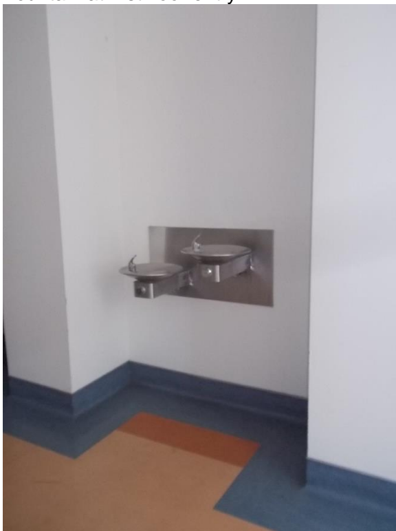
DF3. Compliant DF at second floor SE wing.
