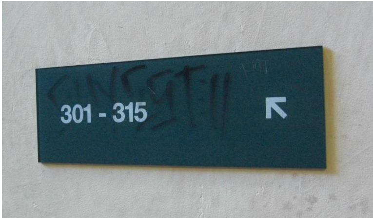
S2. Third floor; wayfinding signage vandalized.
