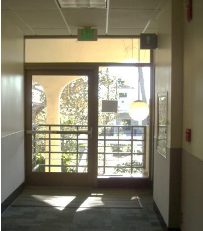
D3. Second floor exit to stairs; tactile exiting signage not provided.
