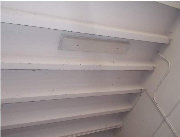
E6. Exterior lighting with surface mounded conduit by elevator.
