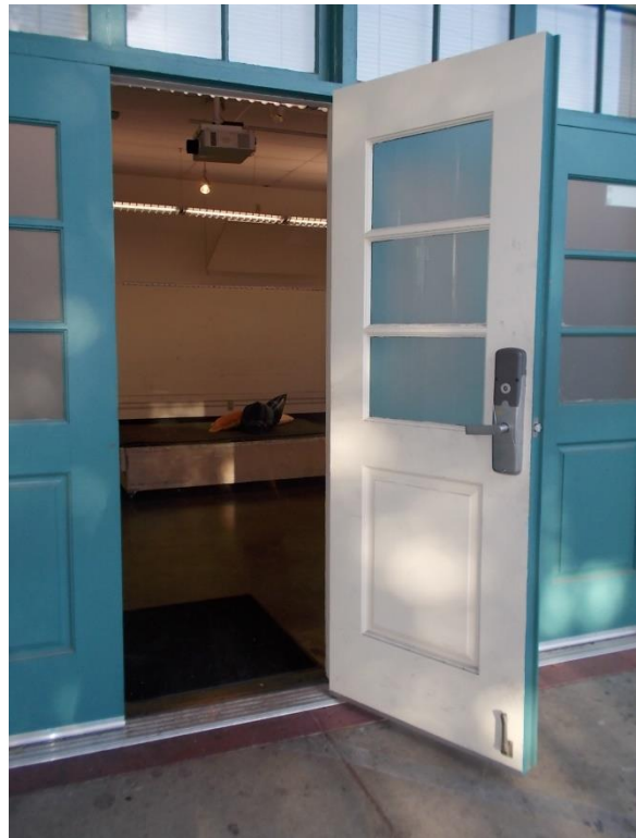
D9. Classroom 23; non-compliant thresholds and no level landing at exit.
