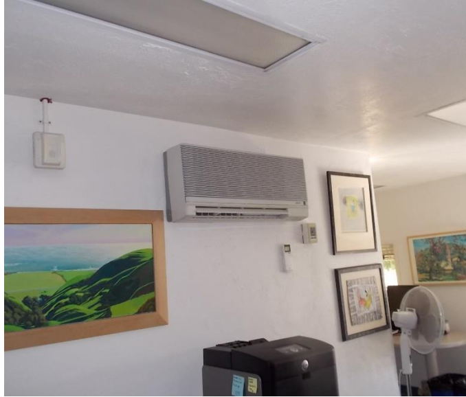
M2. Office 12; wall mounted AC unit.
