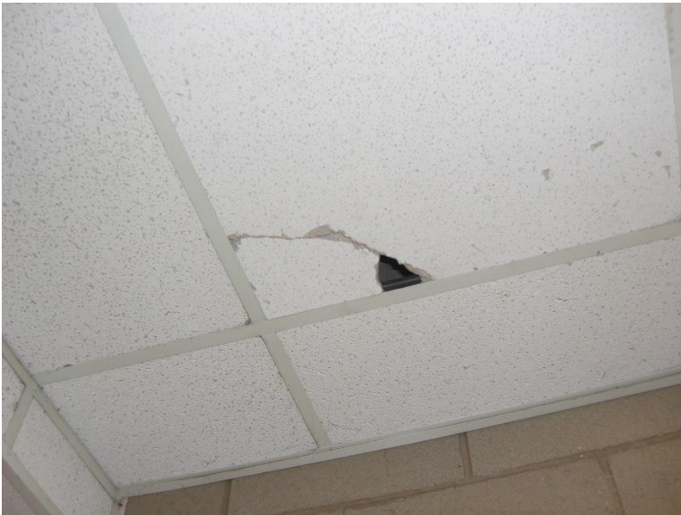
C2. First floor corridor ceiling tile; damaged.
