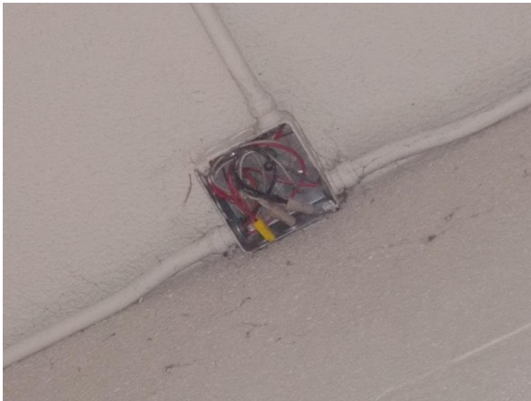
E4. Exposed wiring in j-box.
