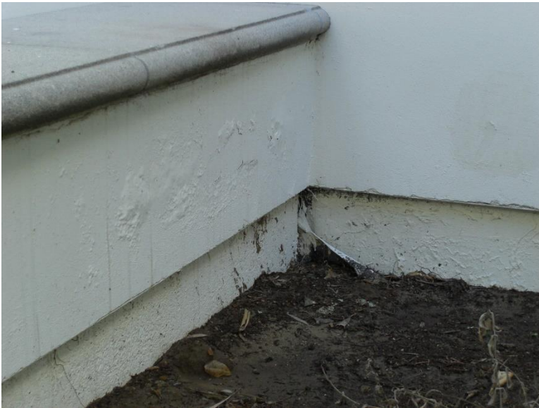
AE2. East exterior wall with bubbling paint.
