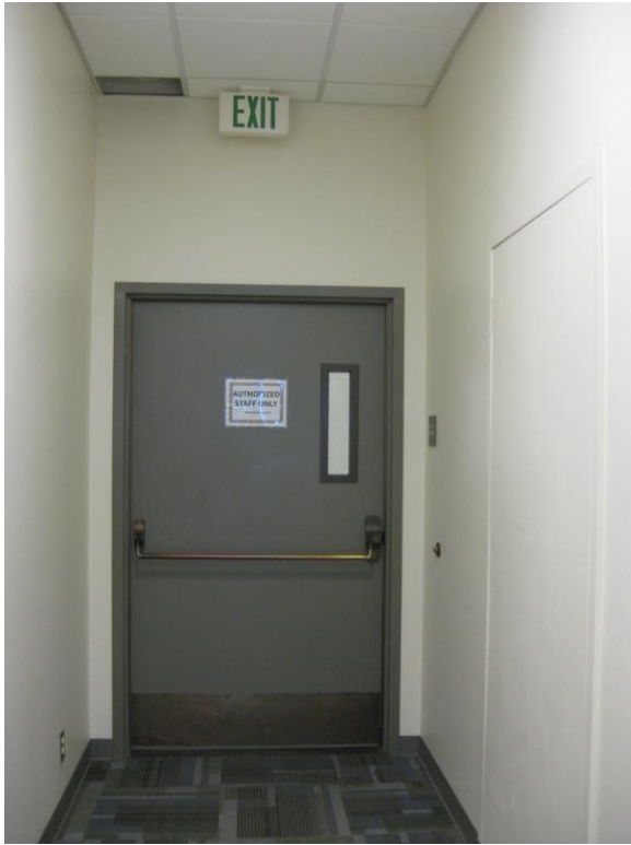
D1. Learning Center area non-compliant exit; side clearance not provided, vision light too high, and exit sign not illuminated.
