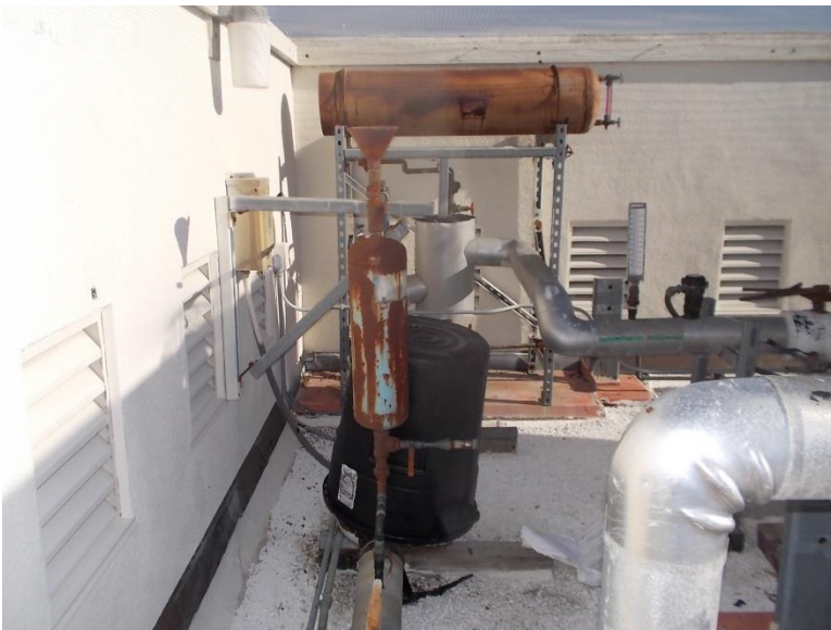
M2. Rooftop mechanical equipment at end of useful life.
