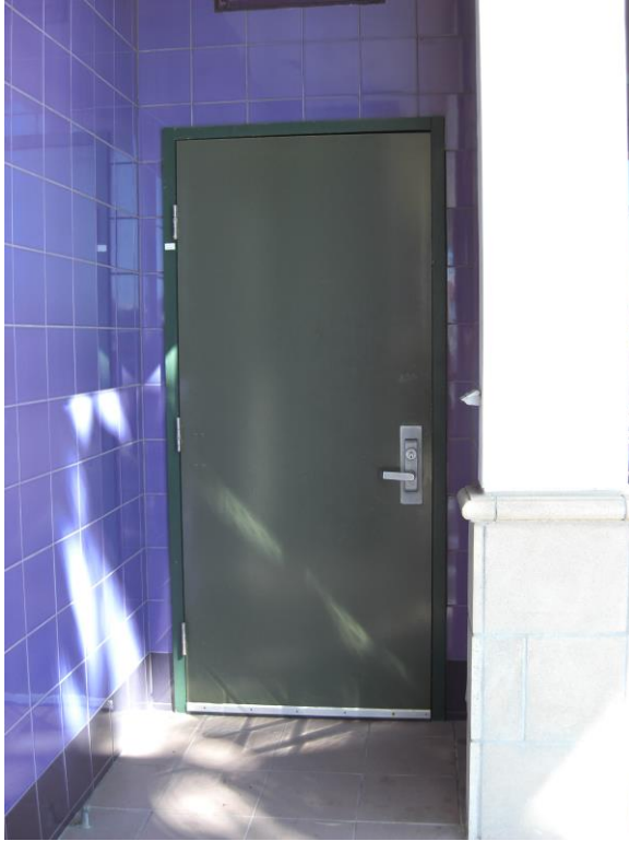
D5. Forum door; non-compliant pull-side clearance, and lacking code required door ID signage.
