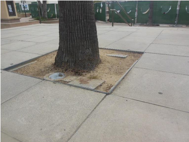
PT4. West entry plaza tree well; hazardous surface feature along path of travel.
