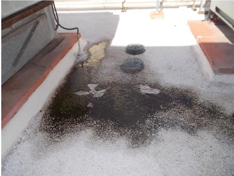
R1. Mechanical roof well with water damage at built up roofing system.
