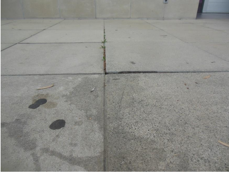
PT3. West entry plaza; abrupt change in level and hazardous surface features along path of travel.
