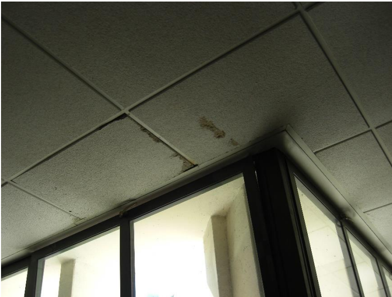
C4. Third floor corridor; damaged ceiling tiles.
