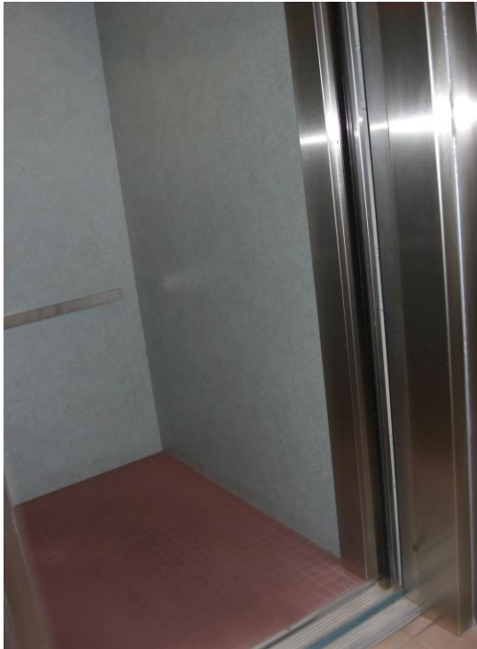
EV1. Elevator access to all floors.
