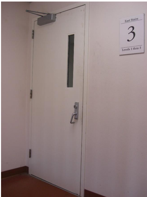
S2. Stairwell exiting signage is inadequate; second floor.
