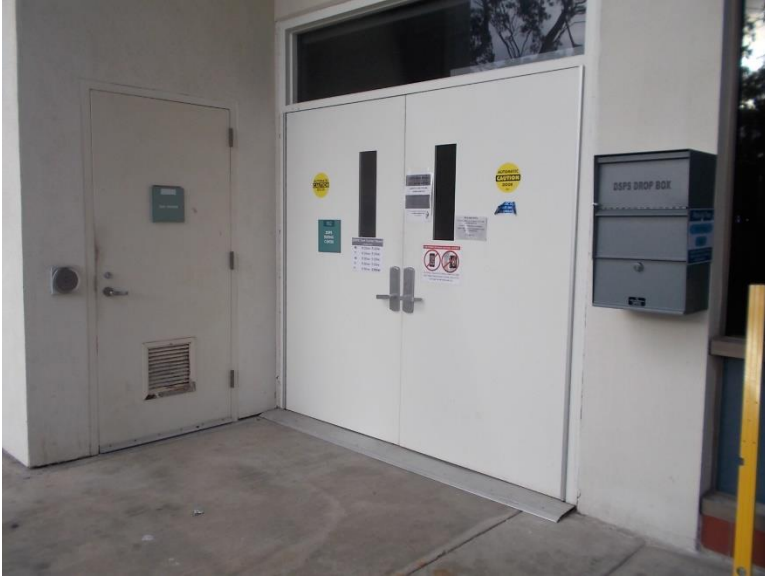
D3. DSPS Testing Lab; non-compliant threshold.
