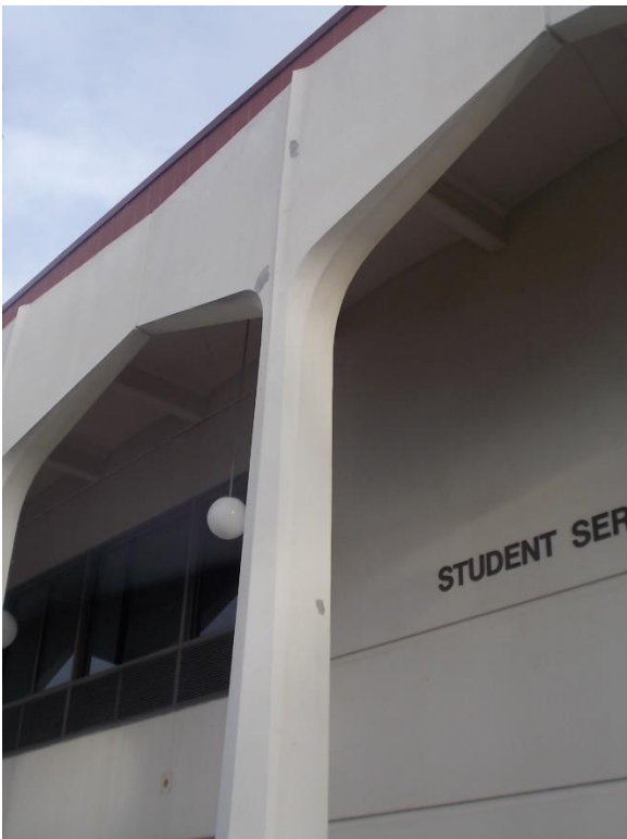
AE2. Exterior walls; peeling plaster paint.
