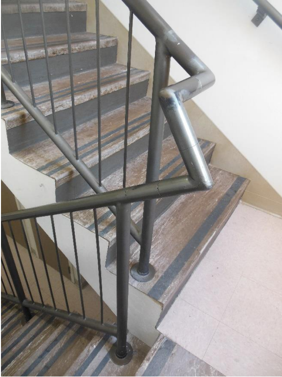
ST3. Stairwell 136; non-compliant handrail heights and returns.
