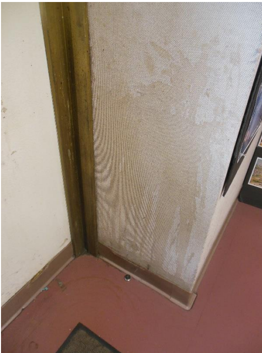
A4. Library vestibule; fabric wallcovering stained.
