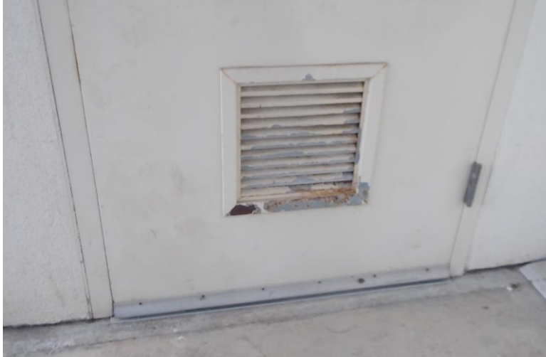
D5. Storage 164 door; damaged louver.
