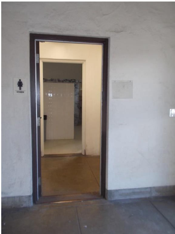
S2. Women's Restroom entrance; room ID signage mounted on wrong side of door
