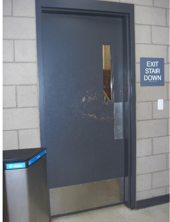
D4. Second floor stairwell door with damaged paint, and no panic hardware.
