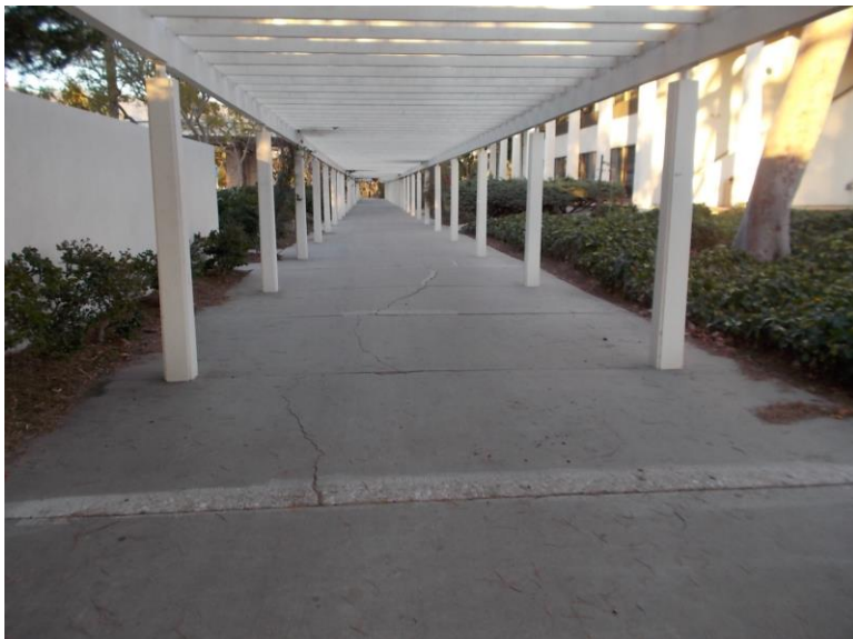
PT2. Exterior walkway Pergola; non-compliant path of travel. Concrete surface is cracked, uneven and has excessive cross slopes. ADA directional signage is not provided.
