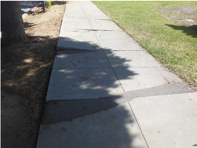
PT10. Public sidewalk at east side of site, near bus stop; abrupt changes in level, and excessive cross slope.
