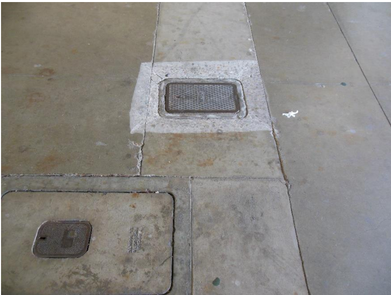
EF4. Exterior corridor walkway; abrupt changes in level.
