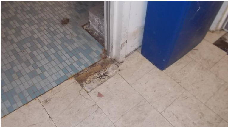
IF4. Basement; 9x9 VAT flooring damage.
