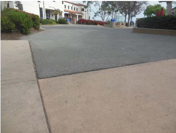
PT9. Northeast exterior walkway; uneven asphalt to concrete transitions. Abrupt change in level and hazardous surface features along path of travel.
