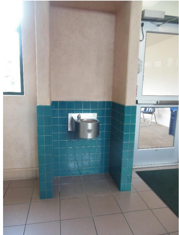
DF2. Third floor; single drinking fountain.
