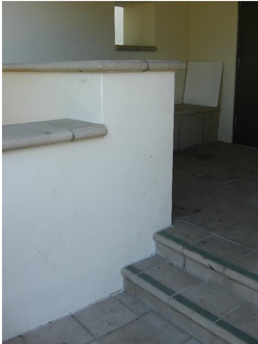
ST1. Exterior north stairs; missing required handrails.
