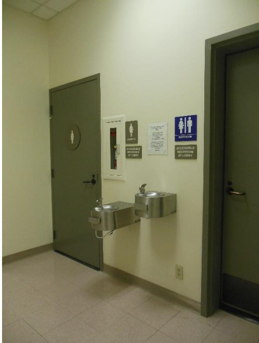
DF3. Corridor 112; non-compliant hi-low drinking fountains.
