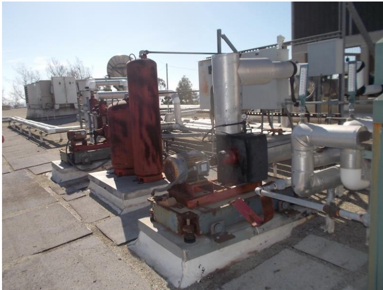
M2. Rooftop mechanical equipment.
