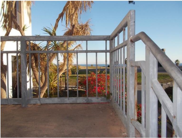
ST1. South exterior stairs with non-compliant and corroded handrails.
