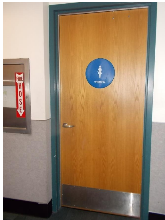
D5. Second floor restroom; push-side clearance not met, wall signage missing.
