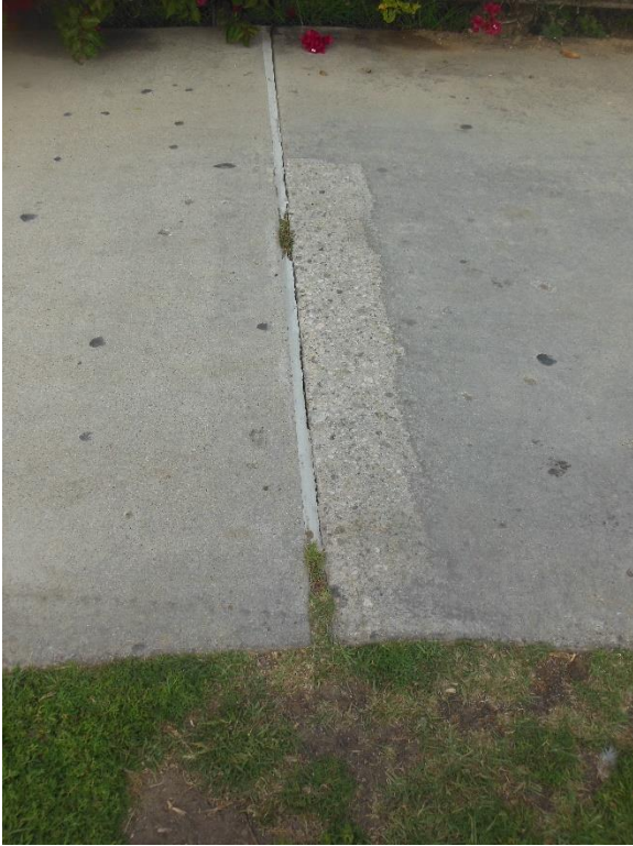
EF3. Concrete walkway, with tripping hazard ground down.
