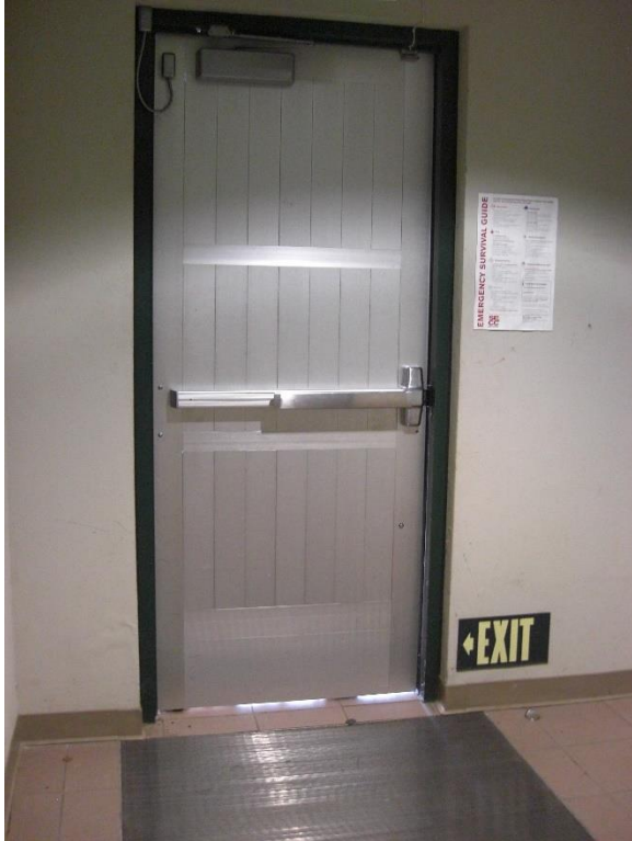
D4. Exit door from Forum lecture hall foyer. Tactile exit sign missing.
