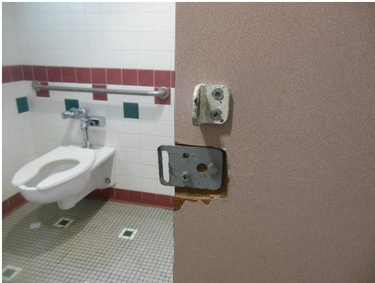
RR6. Café restrooms; damaged accessible stall hardware.
