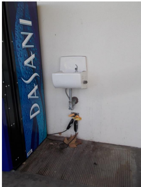
DF4. Non-compliant DF at OE first floor.
