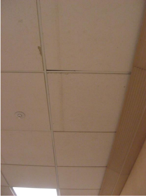
C3. Second floor corridor; damaged ceiling tiles.
