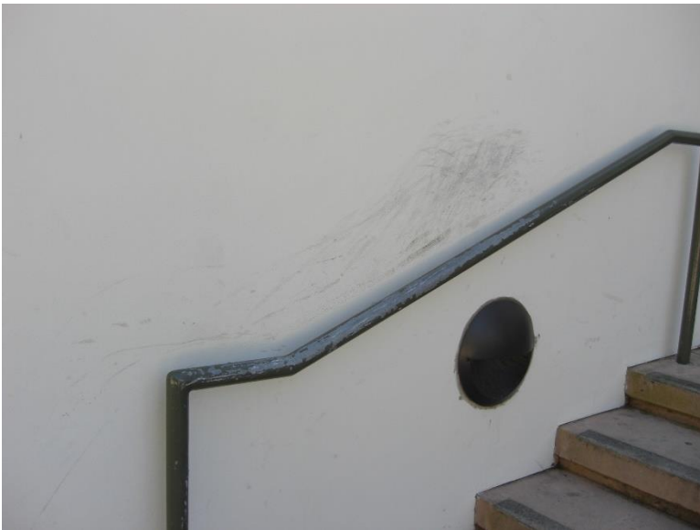
ST6. East side of building; exterior stair handrail finish degraded, and non-compliant height.
