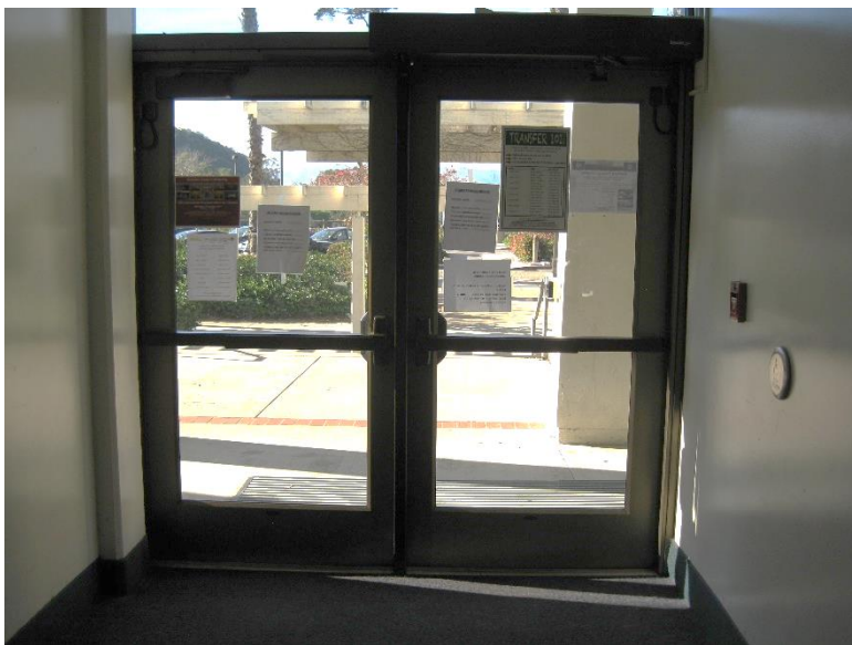
D2. First floor exit; electronic door operator low level access button required by code is not installed, and tactile exit signage not provided.
